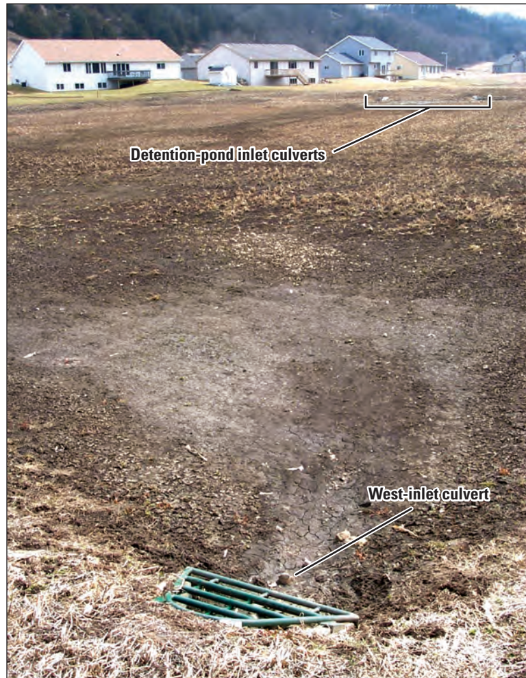
Figure 13. Layer of silt that has formed from excessive ponding of runoff near the west-inlet and main-outlet culverts in the infiltration basin in the low-impact-development basin (April, 2001).
