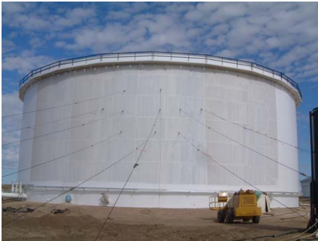
Tank Damaged by Wind (After Pulling Out Dents)
