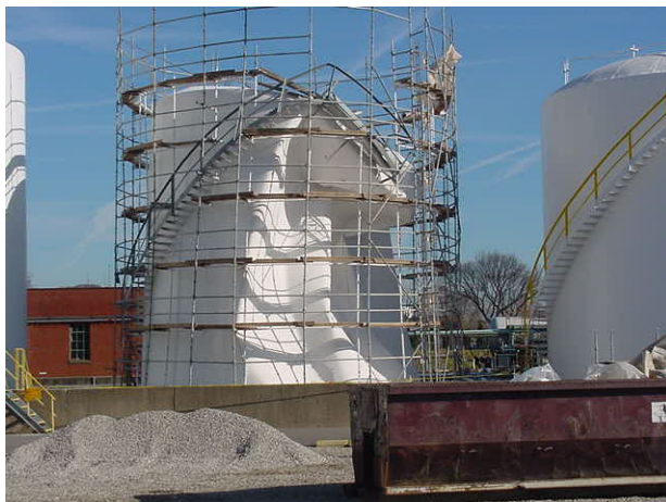
Tank Damaged Beyond Repair by Vacuum
