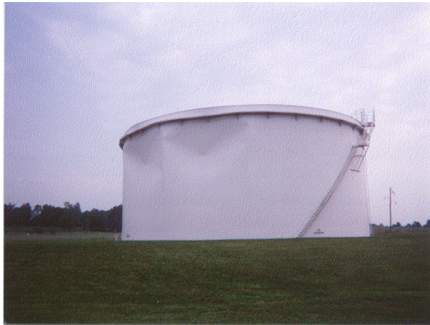
Tank Damaged by Tornado Winds
