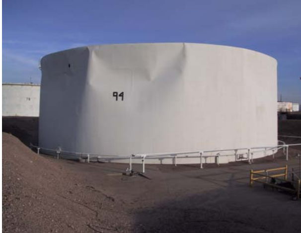
Tank Damaged by Negative Internal Pressure (Vacuum)
