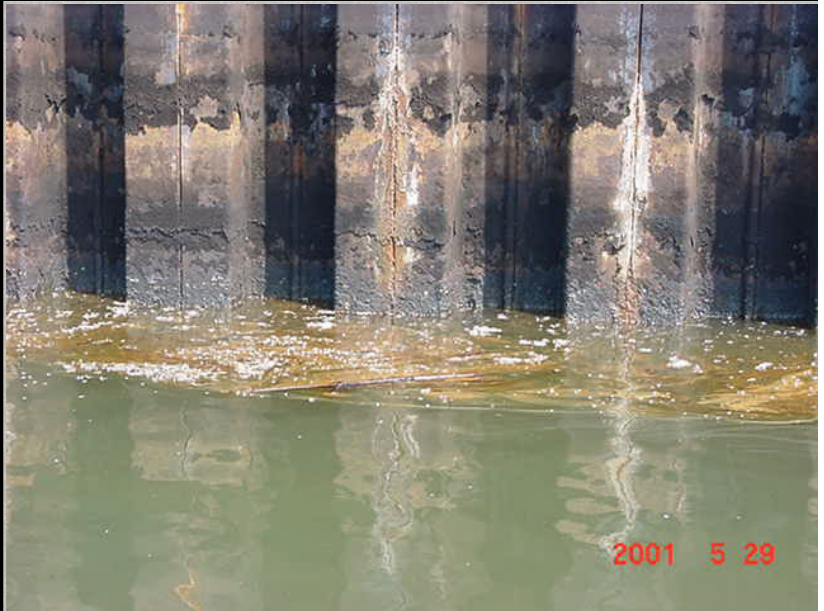
Sheet Piling with Oil Slick
