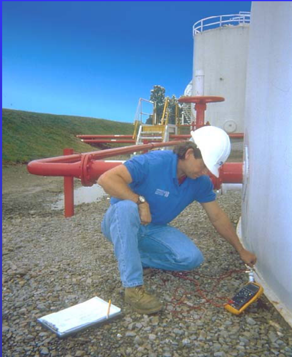
Cathodic Protection Monitoring
