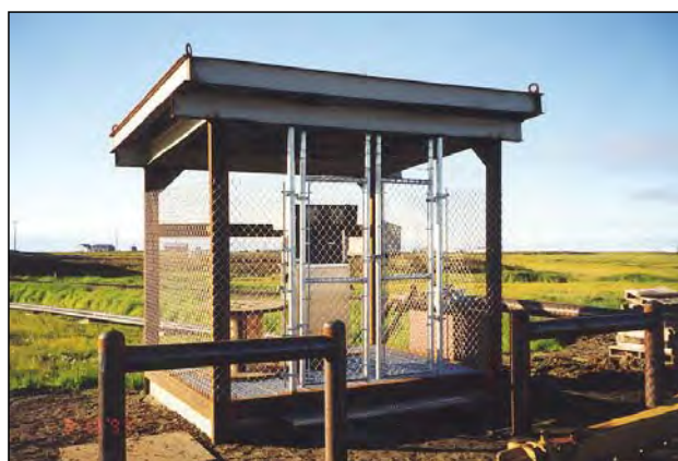
Figure 3-2. Fencing around a dispenser pump.
