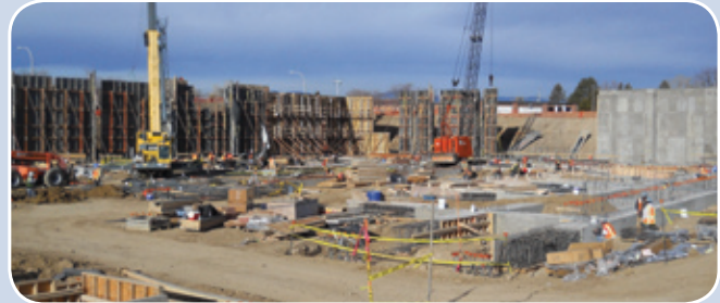
Construction continues on the Department's Enterprise Server Operations Center. State Magazine April 2011
