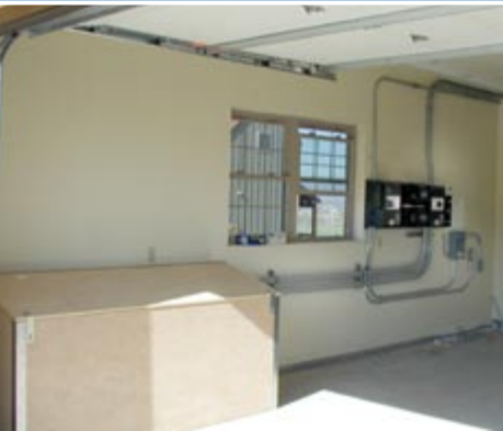
Residential inverter with backup batteries stored inside the box. Photo courtesy of Leif Juell, Alternative Power Enterprises, Inc.
