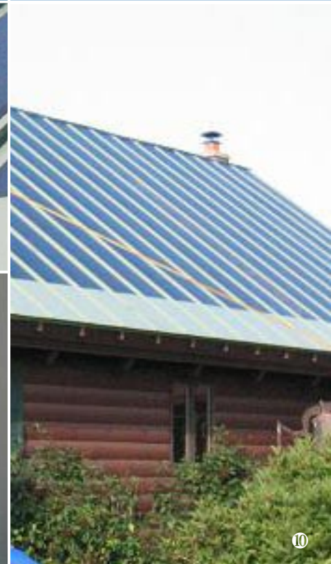
(photo series) Metal standing seam roof laminate systems step-by-step installation. Photo courtesy of Decker Homes.
