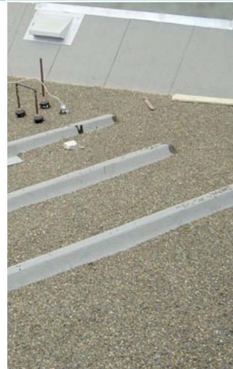
Penetrations through the roof decking are not needed for mounts if curbs are installed as shown on this flat roof.
