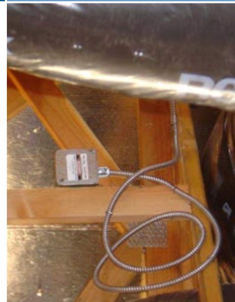
Some BIPV systems tie into a junction box that was installed during the rough-in stage of construction.
