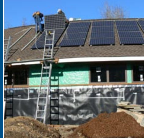
Contractors install PV panels on the curved roof of this custom zero energy home near Olympia, Washington.
