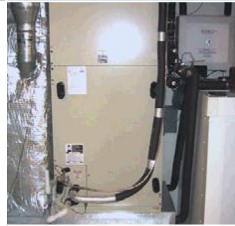
The home's A/C unit (center) and an integrated solar water and space heating system. Solar collectors provide space and water heating with backup heat provided by a tankless water heater (photo from NAHBRC).
