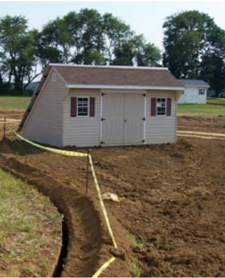
Wiring for the photovoltaic system runs underground from the sheds to the houses.
