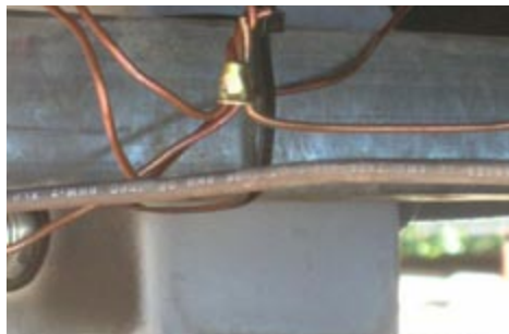
(left) Photo courtesy of John Wiles of SWTDI. (right) Photo courtesy of Kurt Johnson of SunPower
