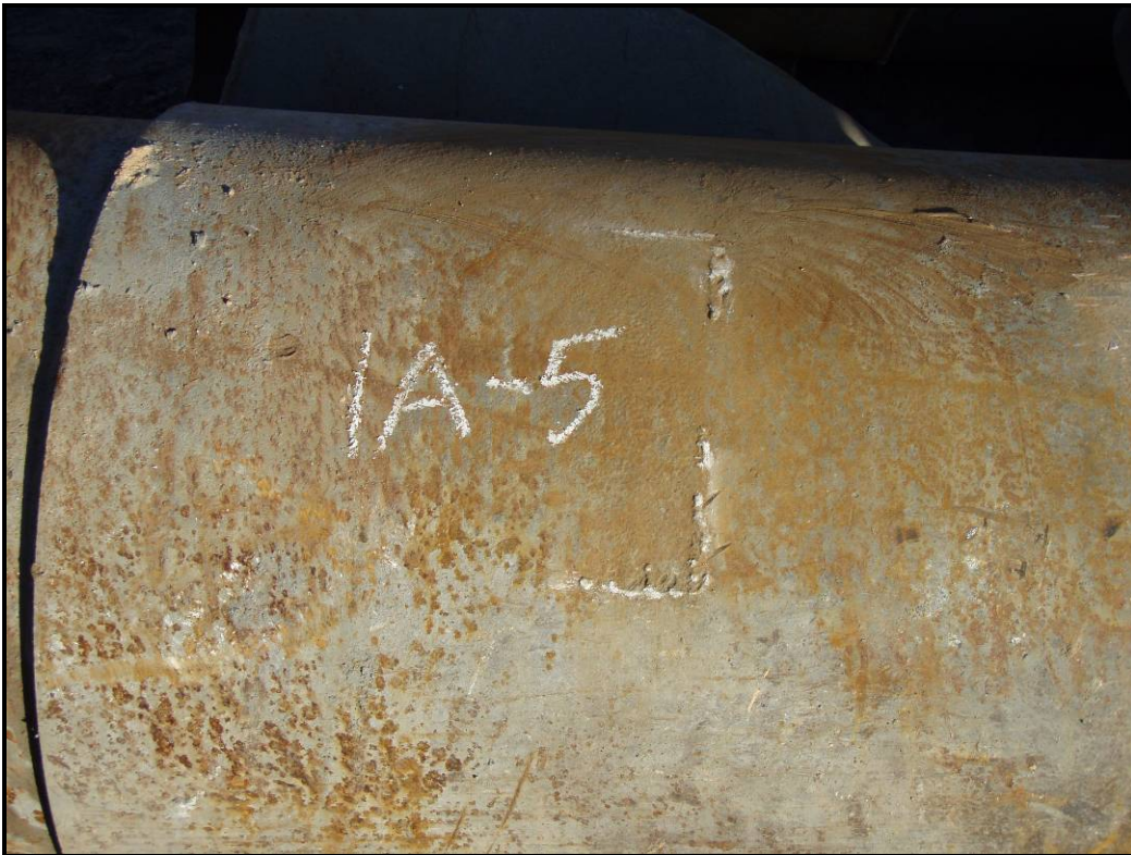
Photo 12 - Minimal bearing plate weld remnant traced in white chalk.
