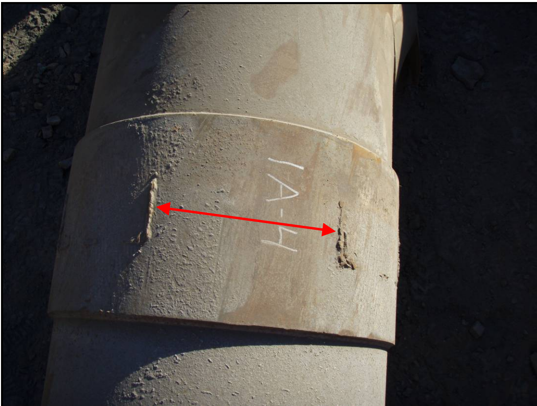
Photo 14 – Weld remnants show the two bearing plates were not installed 180 degrees apart.
