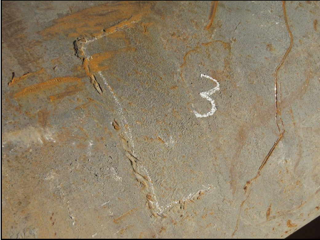
Photo 9 - Minimal bearing plate weld remnant traced in white chalk. Some of weld had been removed.
