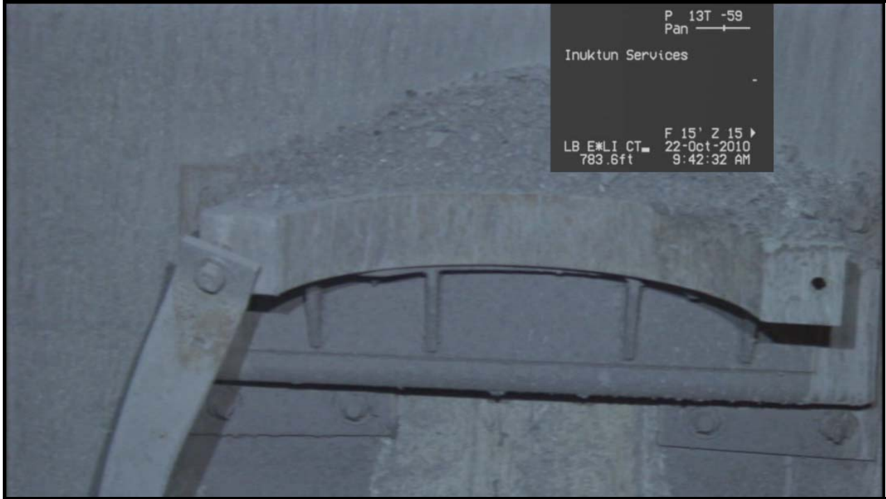
Photo 25 – Video Time 1:57:03 - Single clamp bolt sheared at a new bracket location.
