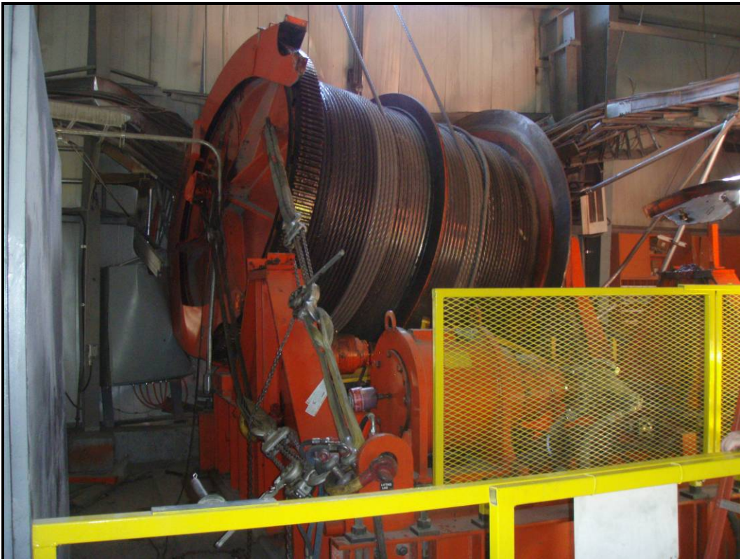
Photo 4 – Ventilation shaft hoist drum ripped from pillow block mounts.
