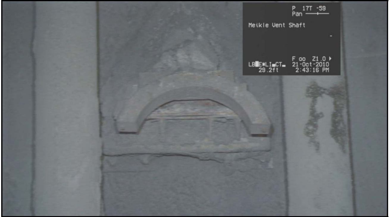
Photo 17 – Video Time 3:31 - Clamp bracket tilted downward and both clamp bolts sheared at a new bracket location.
