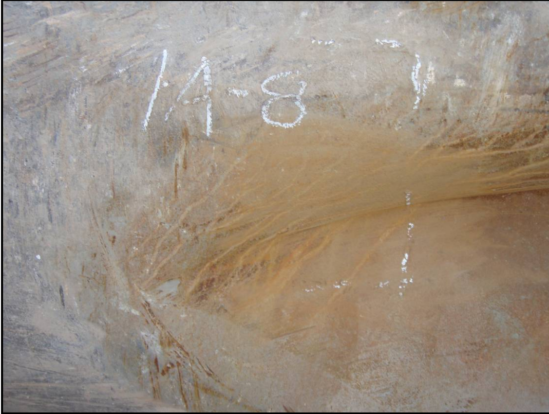
Photo 13 – Minimal bearing plate weld remnant traced in white chalk
