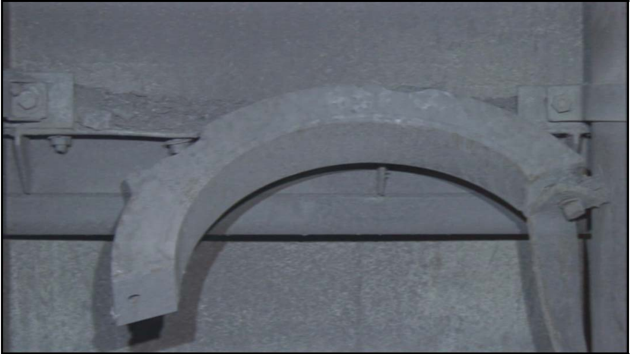
Photo 23 – Video Time 1:15:02 - Original bracket with one clamp bolt failed and a clamp bracket tilted down.
