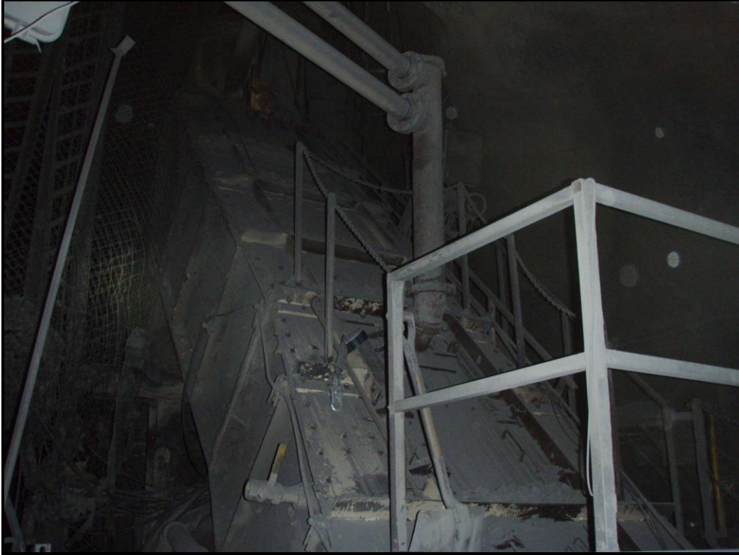
Photo 3 – Discharge chute leading from side of rock box at 860 level.
