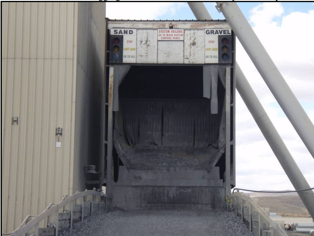
Photo 2 – Surface feed grizzly and hopper adjacent to top of ventilation shaft. Note stop and go operation lights above the hopper.
