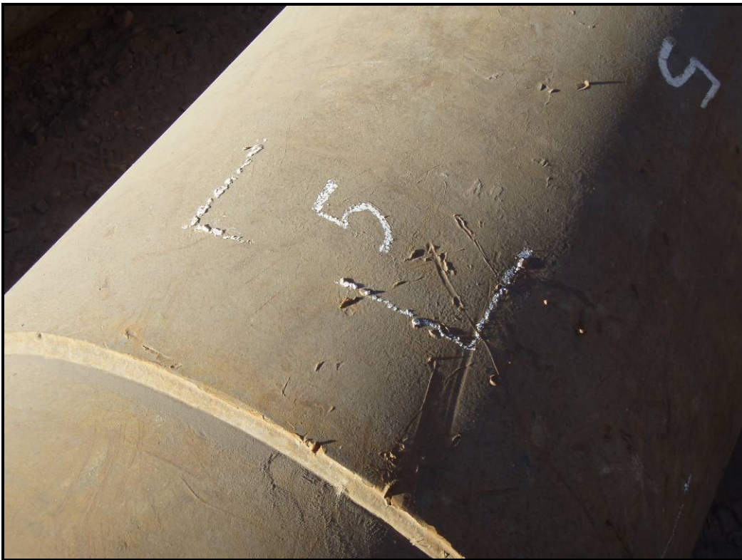
Photo 10 - Minimal bearing plate weld remnant traced in white chalk.
