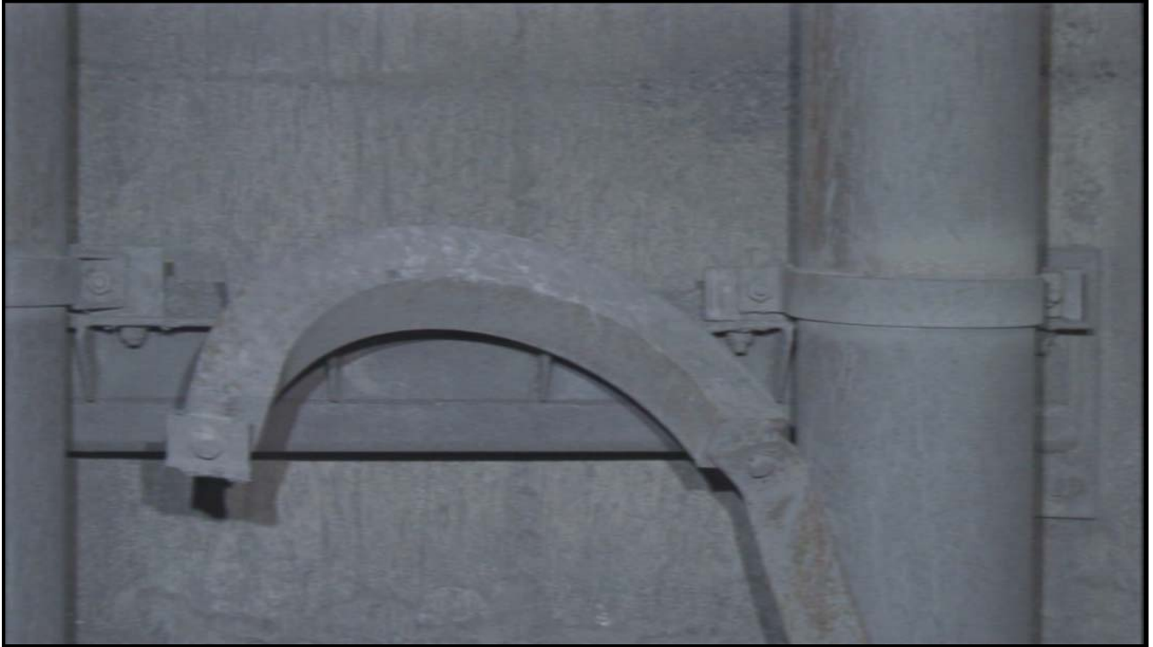
Photo 21 – Video Time 1:05:33 - Sheared clamp at an original bracket location. The clamp bracket was also tilted down.
