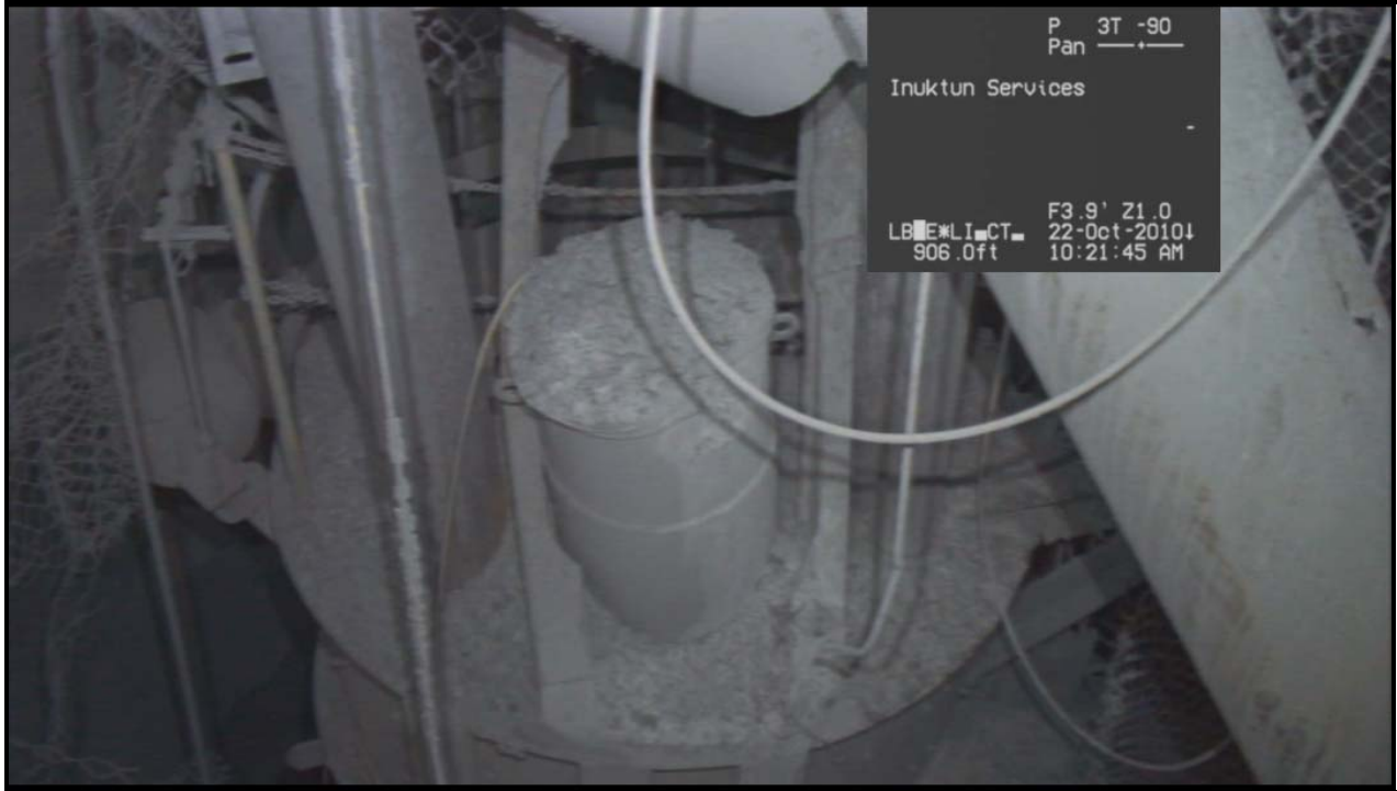
Photo 27 – Video Time 2:36:14 – 860 level rock box (silo) with lowest spool of 24-inch-diameter pipe sticking out of the top. The pipe was filled with aggregate and had dropped into the box.
