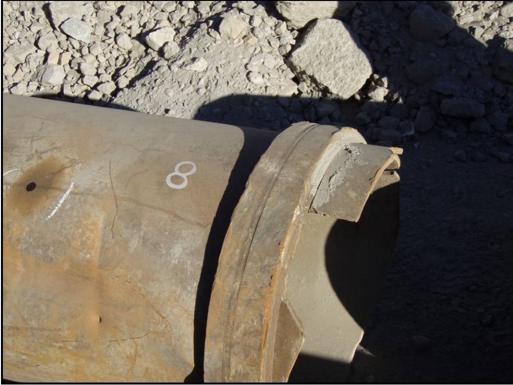
Photo 7 – Two pipe spools welded together in lieu of using a Victualic coupling.
