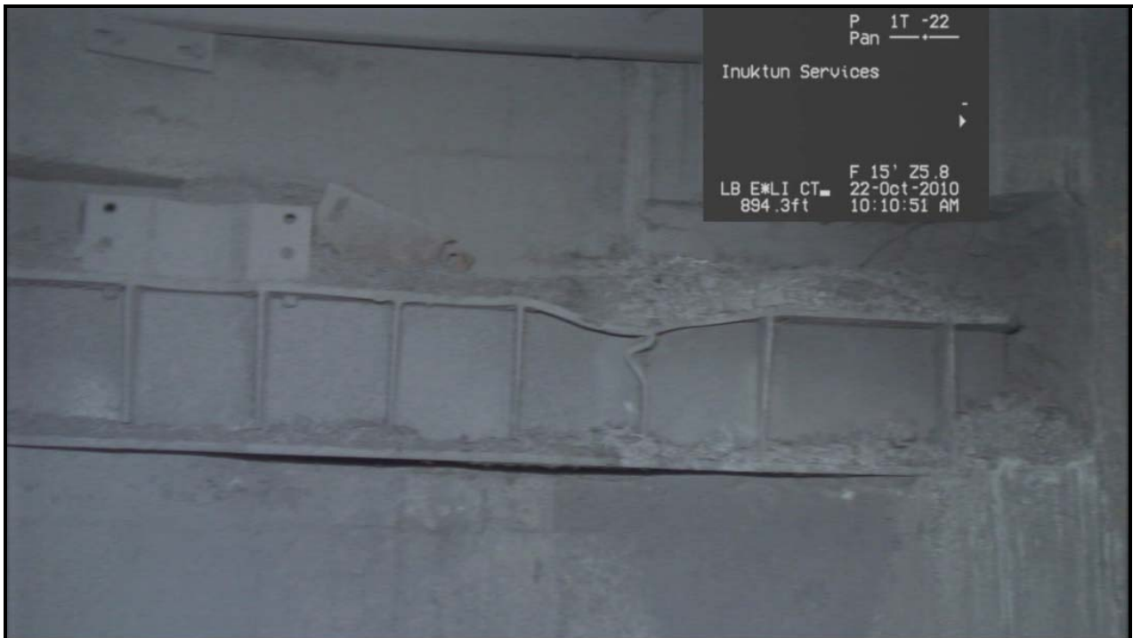
Photo 26 – Video Time 2:25:22 - Lowest bearing bracket with buckled stiffener where a 12-inch diameter pipe was previously attached. The bracket was at shaft elevation 807.
