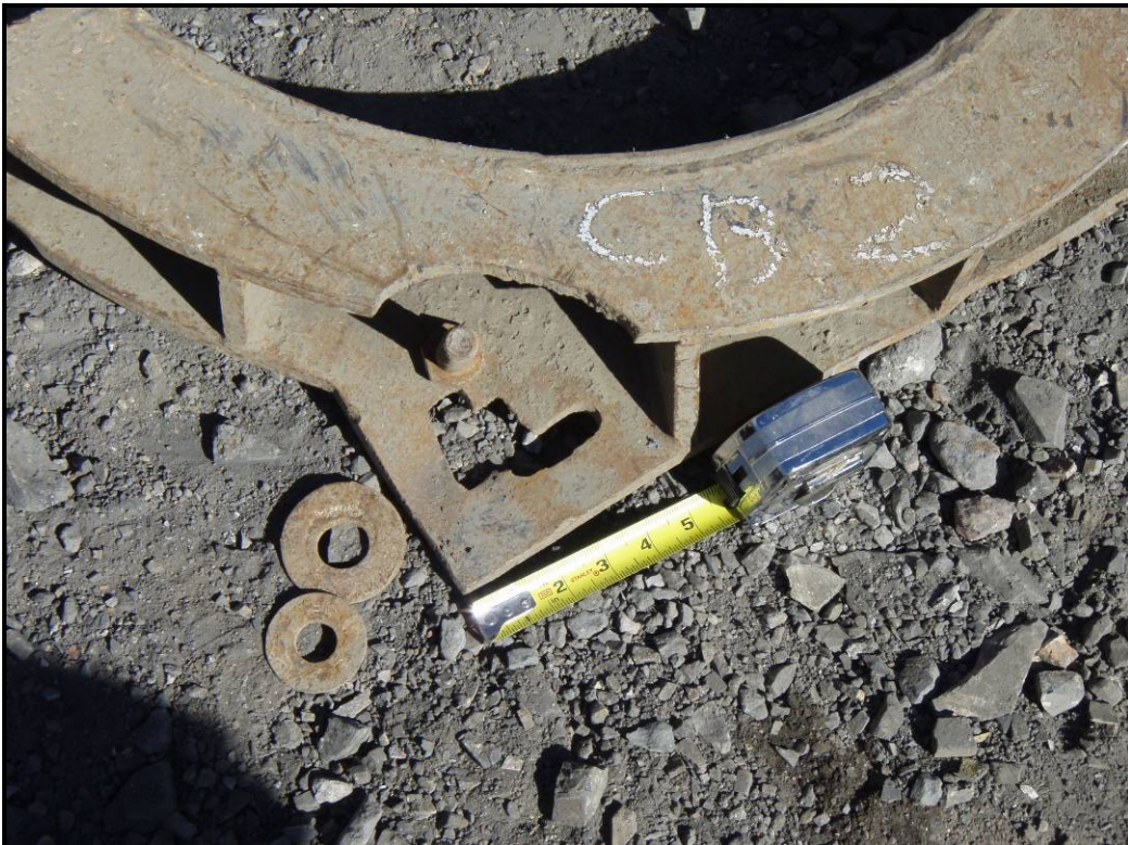
Photo 8 – Slotted hole for A325 bolt used to attach clamp bracket to bracket. Slot was burned out and was larger than the bolt head. This connection would have required a large washer.
