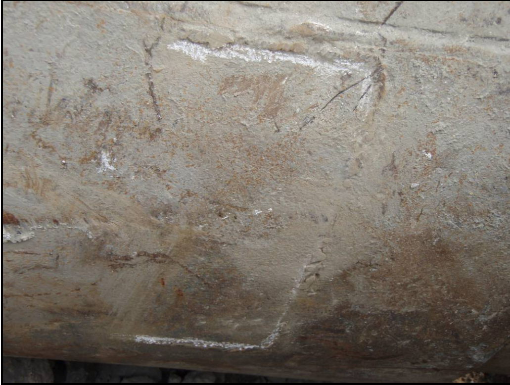
Photo 11 - Minimal bearing plate weld remnant traced in white chalk. Some of weld had been removed.
