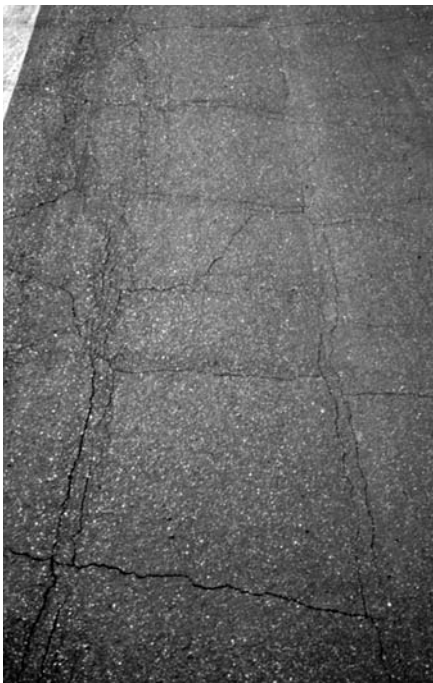
▲ Block cracking with cracks less than 5' apart.
