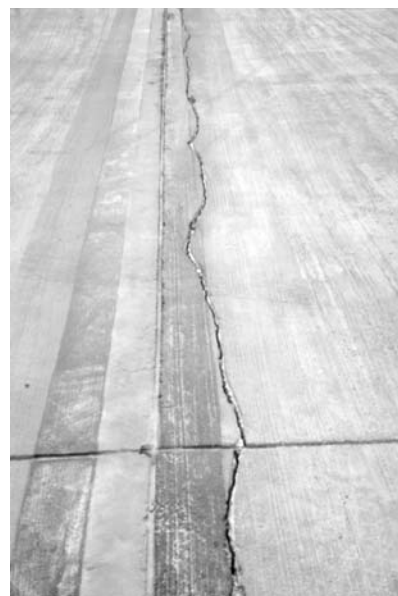
◀ Crack parallel to joint. Open 1/4". No spalling.
