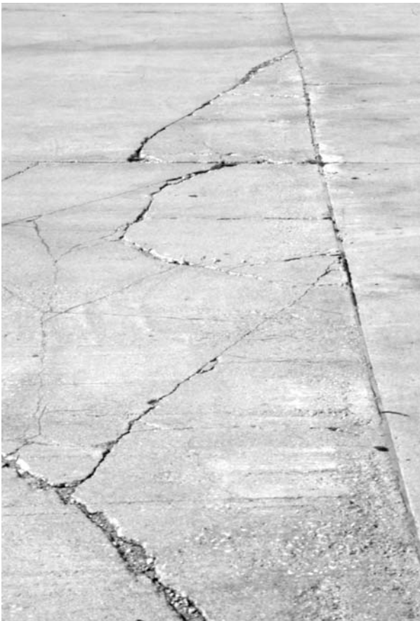
▲ Multiple slab cracks, spalling and shattered slabs.
