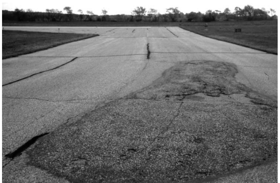
▶ Patch in poor condition.
