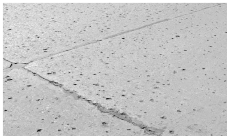
► Extensive pop-outs of large aggregate from surface.
