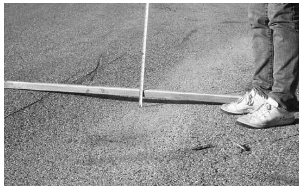
▲ Severe settling from utility trench.
