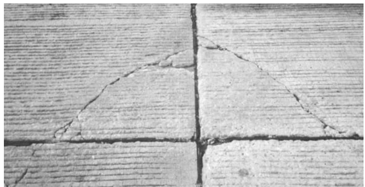
Corner cracking with slight spalling.
