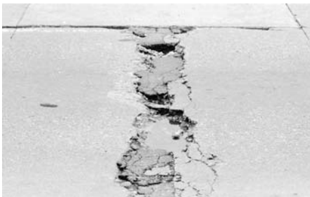
▼ Potholes caused by severe joint deterioration. Need repair.
