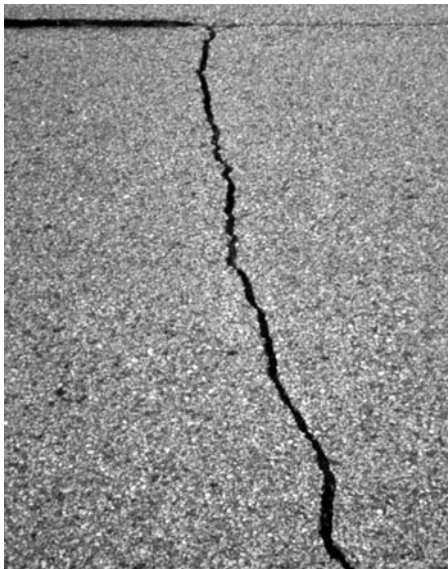
▼ Open cracks need sealing.
