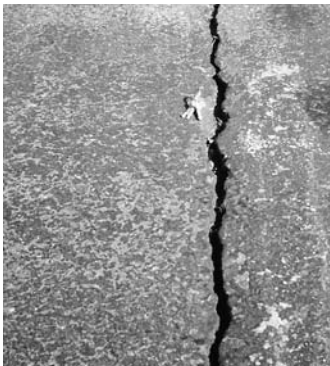
▲ Open crack – 1/2" or more in width.
