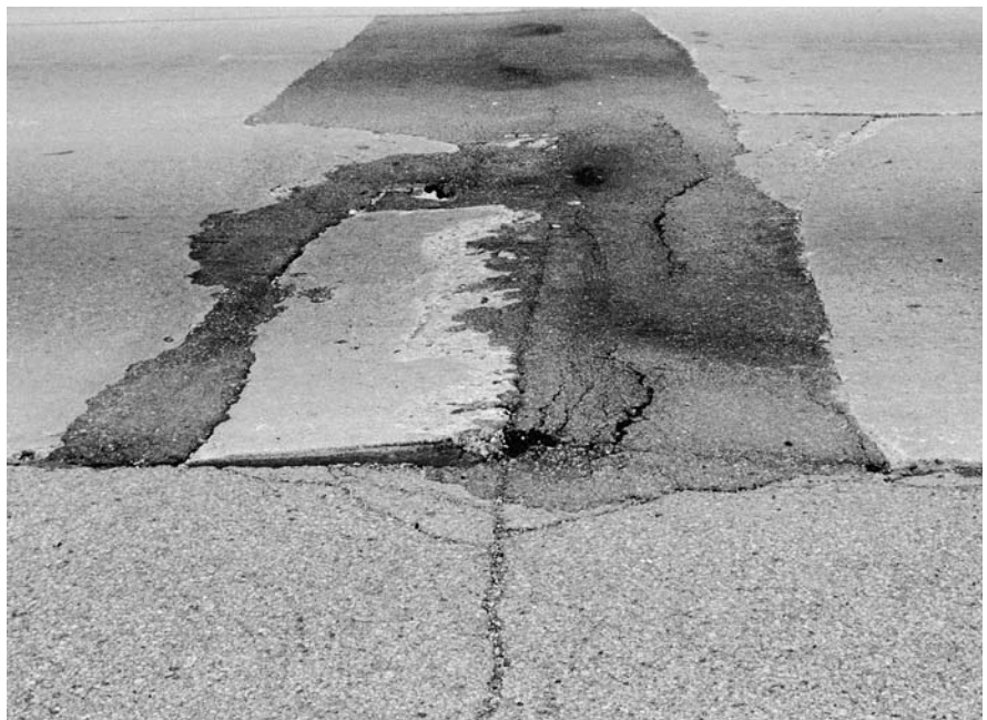
▲ Internal pressure has partially raised slab at the joint. Complete replacement is required.
