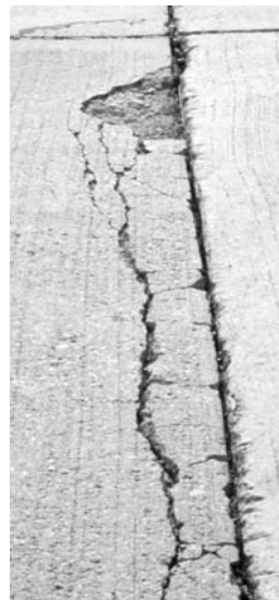
▲ Full depth joint repair required.
