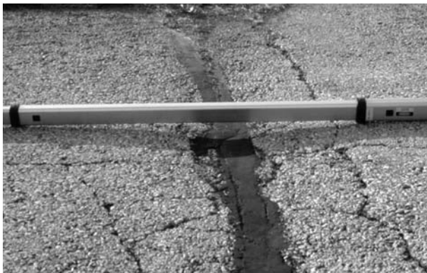
Significant settlement (over 2") and cracking adjacent to sealed crack.
