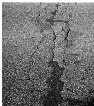
▲ Water enters unsealed cracks softening pavement and causing secondary cracks.
