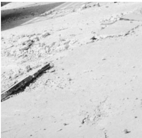
▼ Pavement blowup in progress—concrete is crushed and slab buckled.
