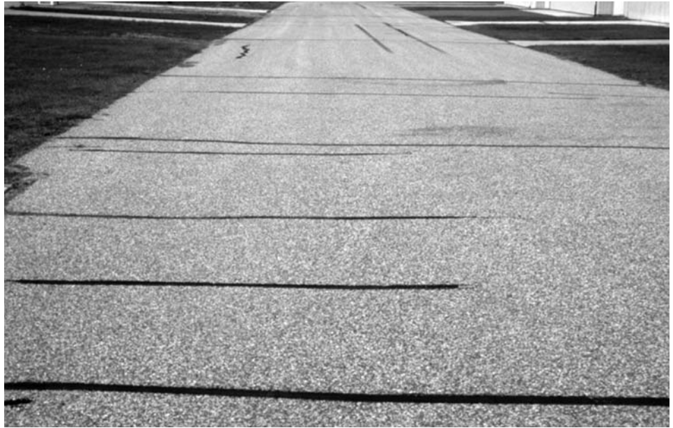
▲ Thermal cracks less than 10' apart. Slight raveling.
