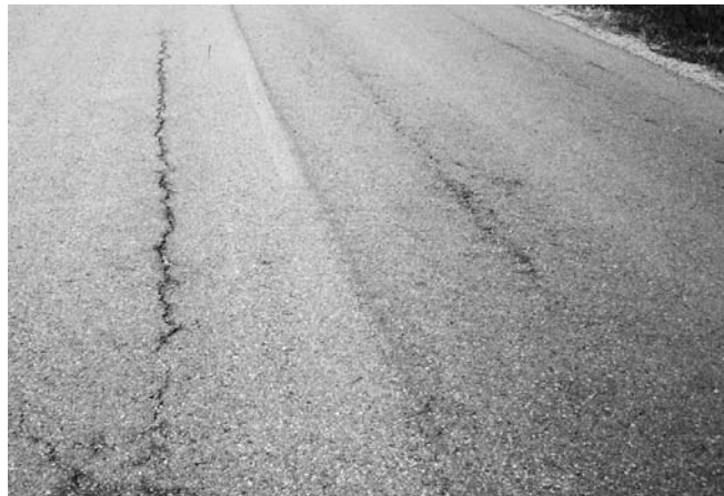
◀ Partially open 1/4" paving joint.
