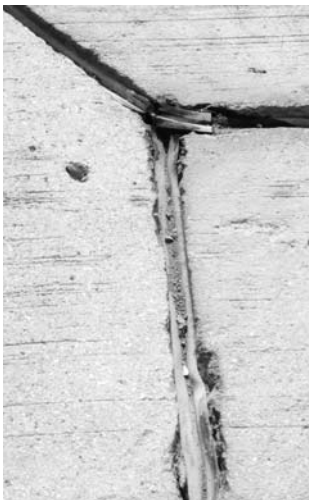
▲ Joint sealant in poor condition. Loss of bond to edge allows water into pavement.
