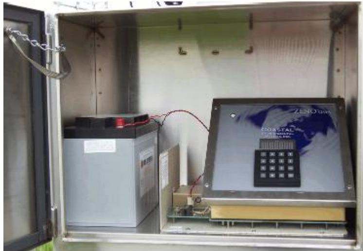
Figure A-16. Data Logger Box
