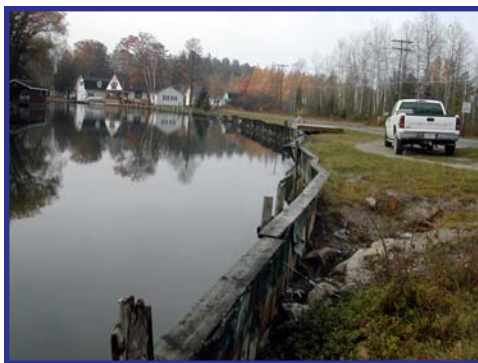
-USFWS photo by Heather Rawlings Aging steel seawalls define this small riparian property in Indian River, Michigan. The Greendocks project will restore this site at both the in-stream and riparian levels for both community and natural resource use.
