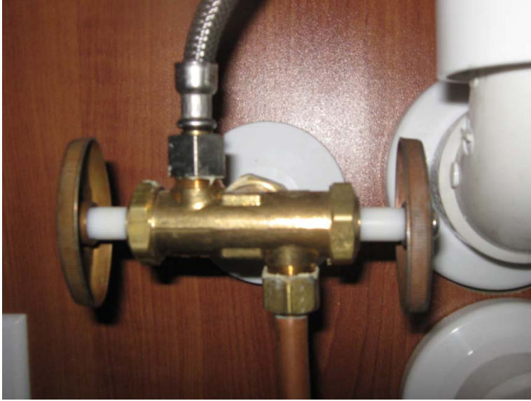
An example of the copper plumbing.
