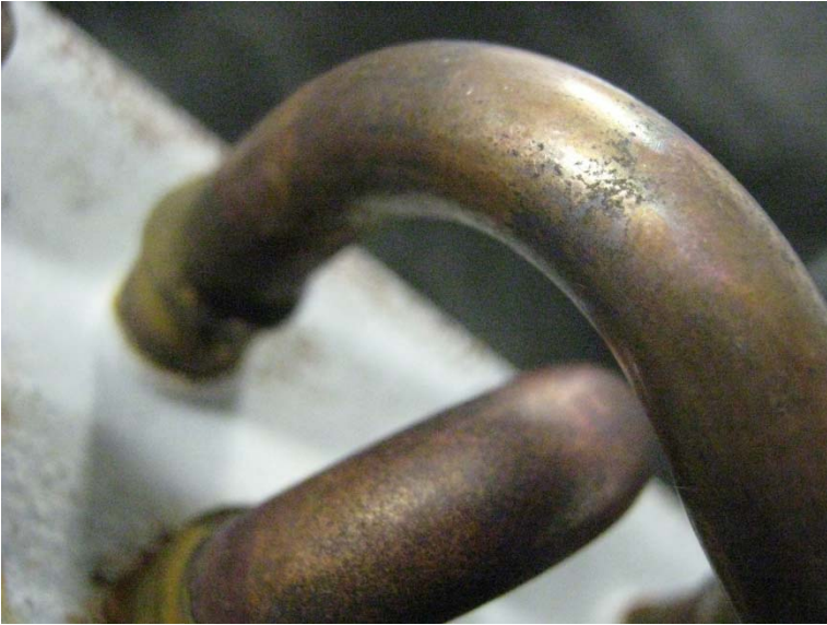
Close-up of AHU coils.
