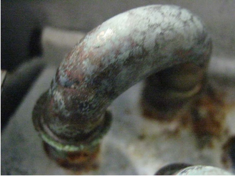
Close-up of AHU coils.
