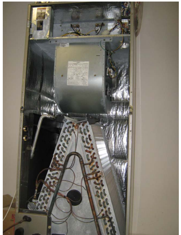
The air-handler unit within the garage.
