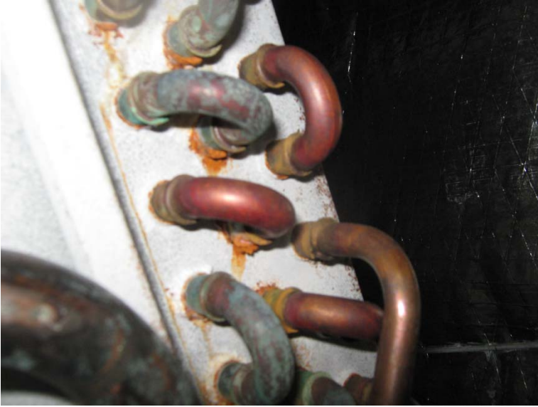
Close-up of AHU coils.
