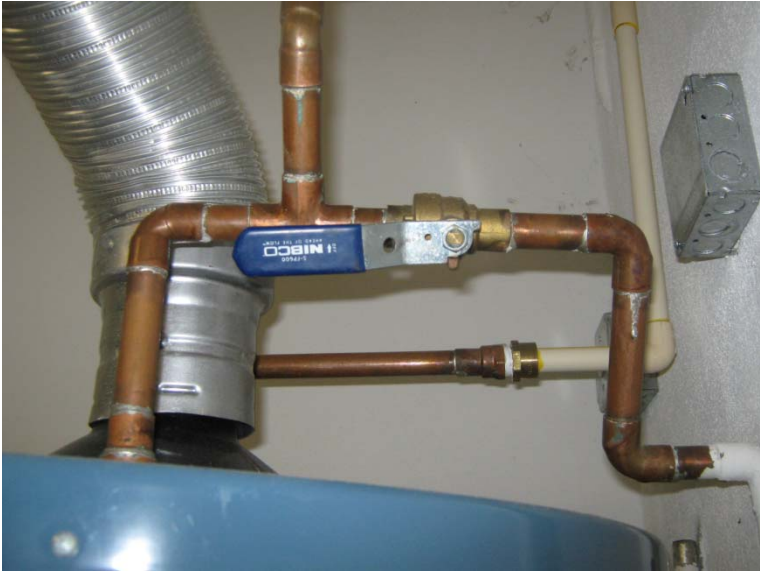
An example of the copper plumbing.
