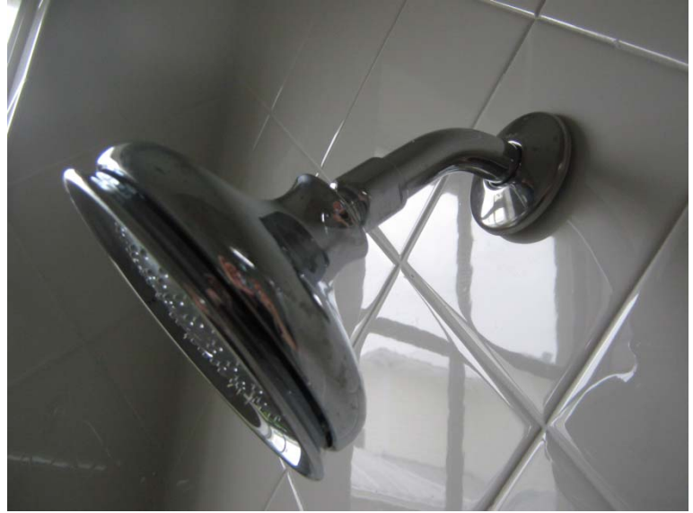
An example of the plumbing fixtures.
