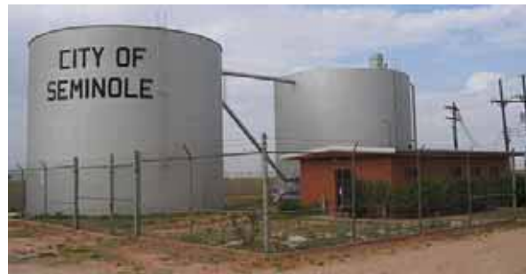
Figure 3.3. Settling Tanks at Seminole Wellfield
