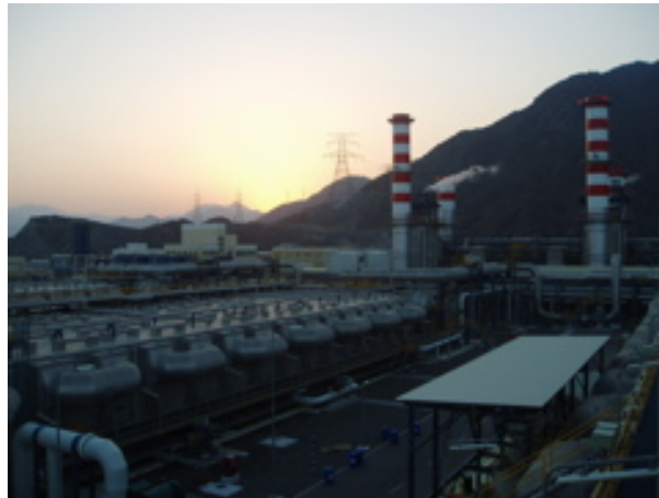
Figure 8. Fujairah, UAE Hybrid Cogeneration – 650 MW 300,000 m 3 /d MSF and 170,000 m 3 /d SWRO.
