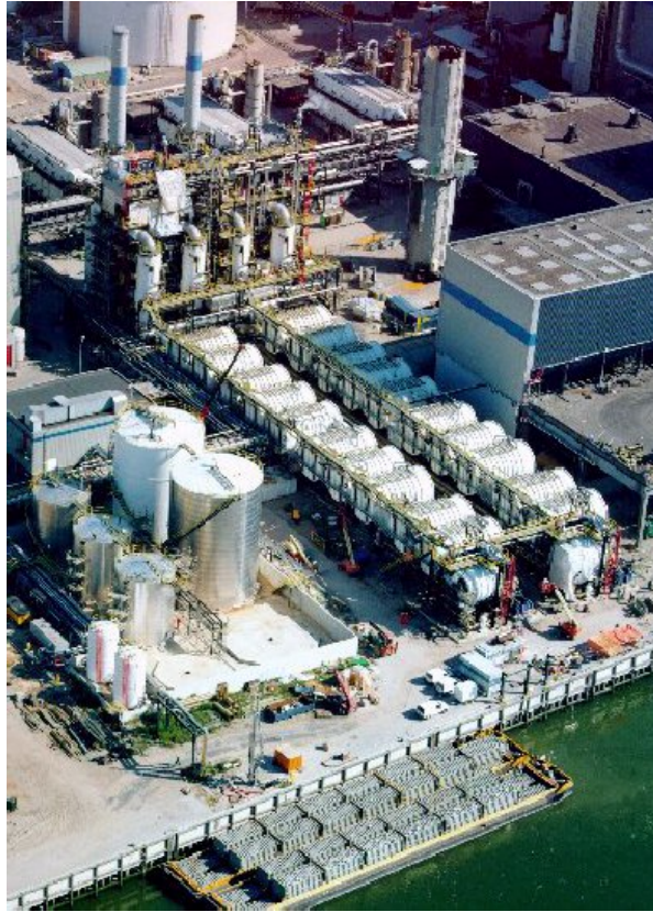
Figure 7. AVR Rotterdam Waste Incinerator 2 x 12,000 m 3 /d/ MED Units (Photo Courtesy Magy Al-Allawy).
