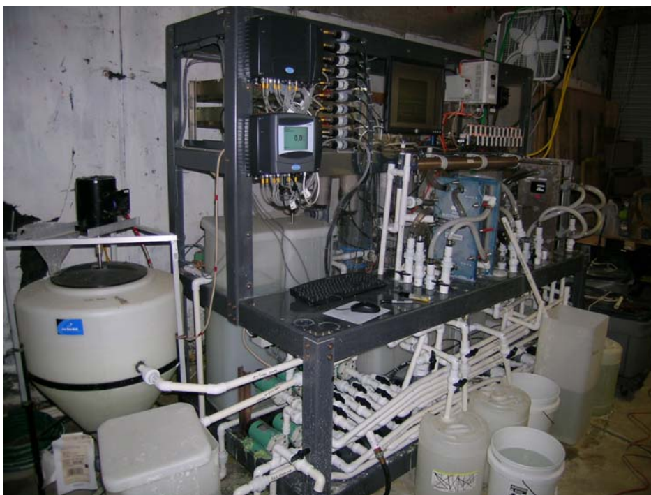
Figure 5. ZDD pilot skid installed at Panoche farm.
