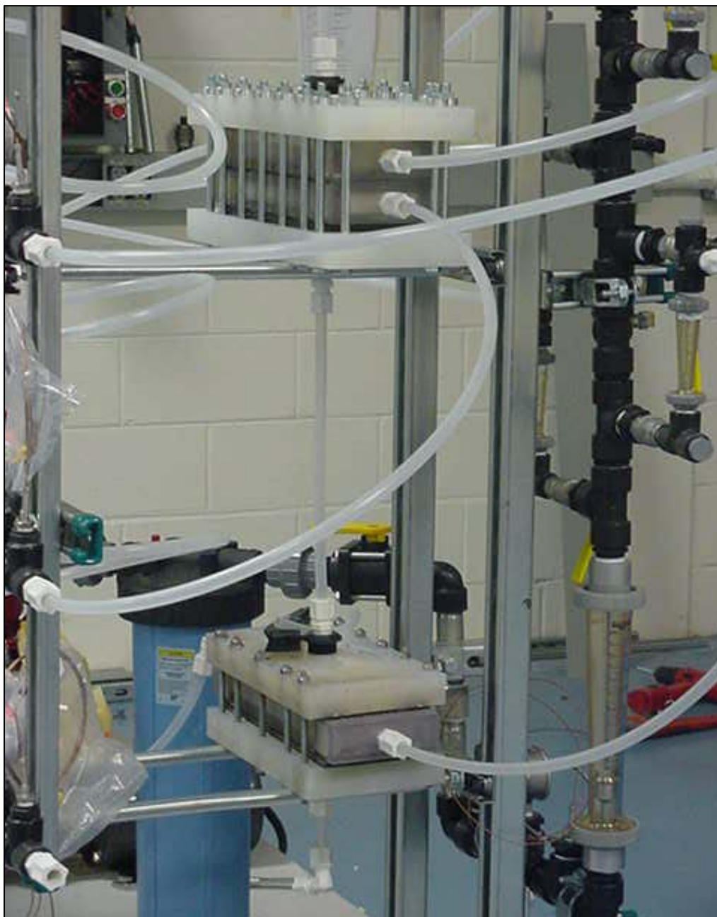
Figure 12c. Photograph of the membrane module assembled in DCMD pilot-scale demo system.
