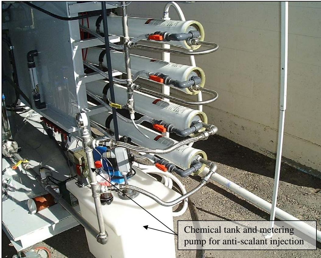
Figure 3-3. Chemical injection system.
