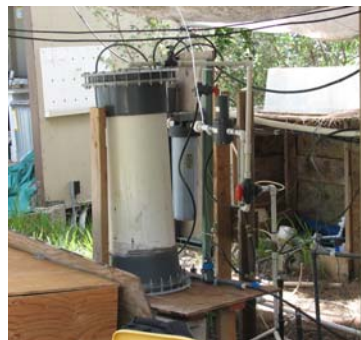
Figure 20. Carbon Filter of Feed Water Pretreatment.
