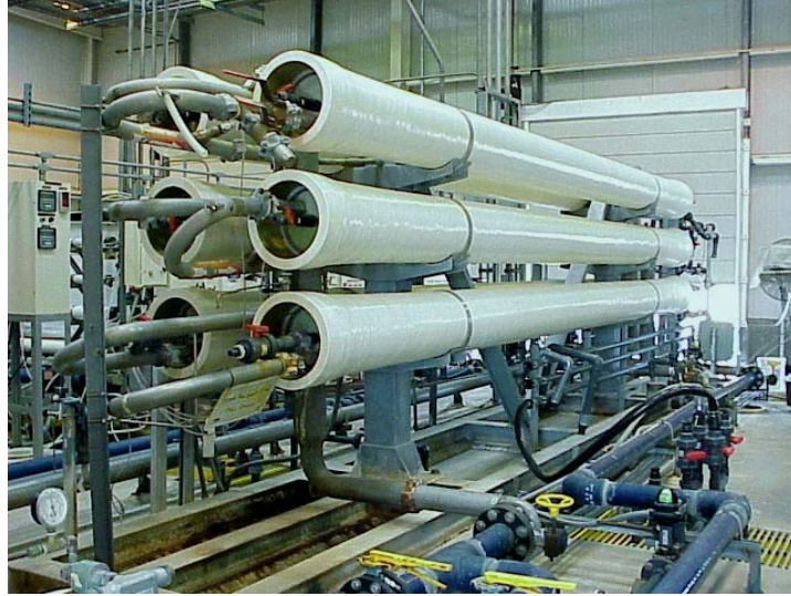
Photo 5.—Fluid Systems Reverse Osmosis Unit.
