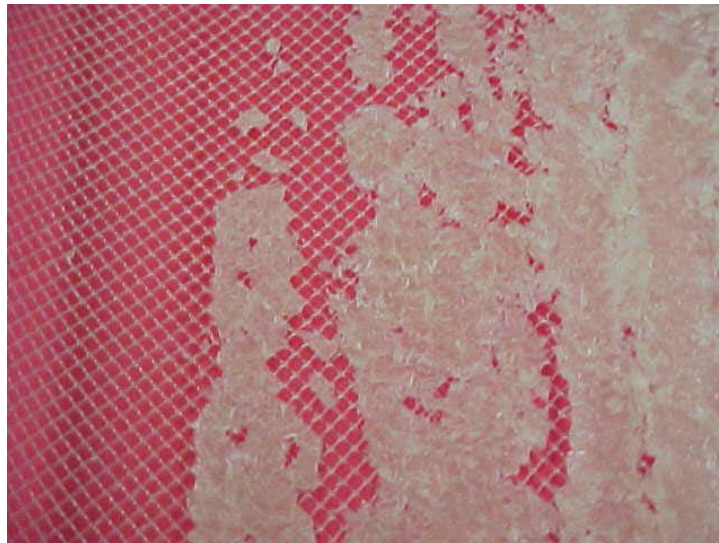
Photo 10.—Calcium Sulfate Scaling - HVC Installed on MU 1 Interstage.
