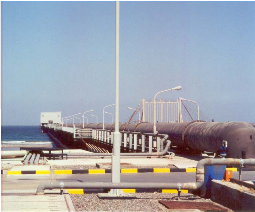
Figure 2-5 Ghubrah Complex seawater intake lines
