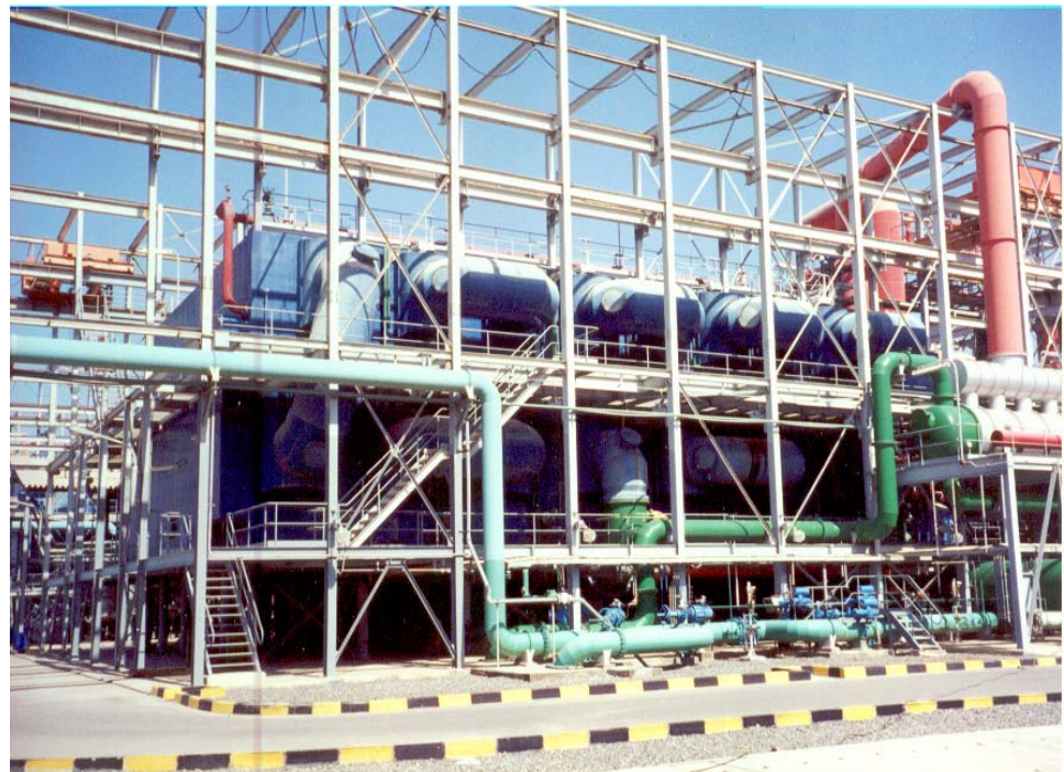
Figure 2-6 MSF unit at the Ghubrah Complex
