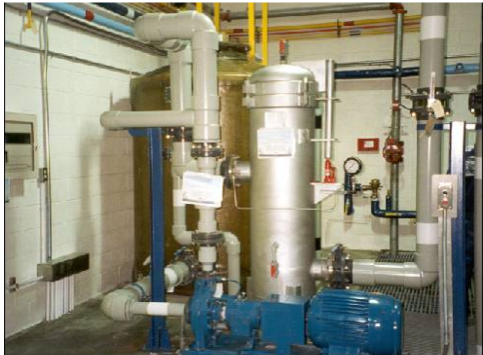
Figure 4-40 Cleaning system, North Hatteras plant, Dare County, North Carolina
