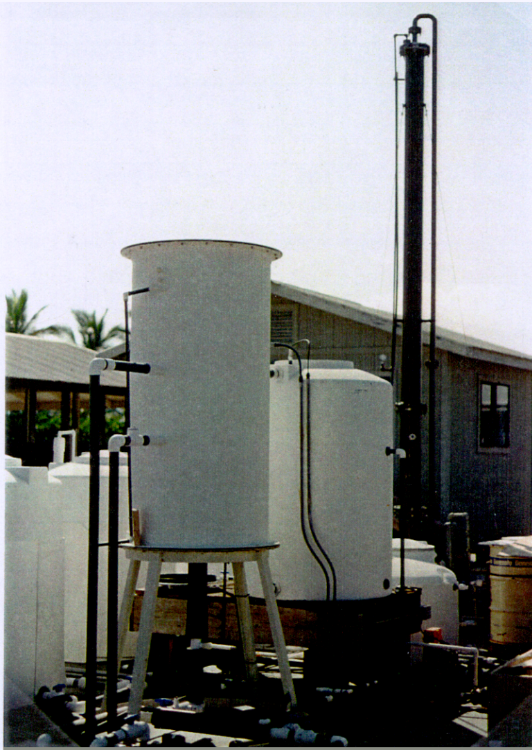
Figure 5-9: Wash Column, Product Water Tank and Vacuum Tower
