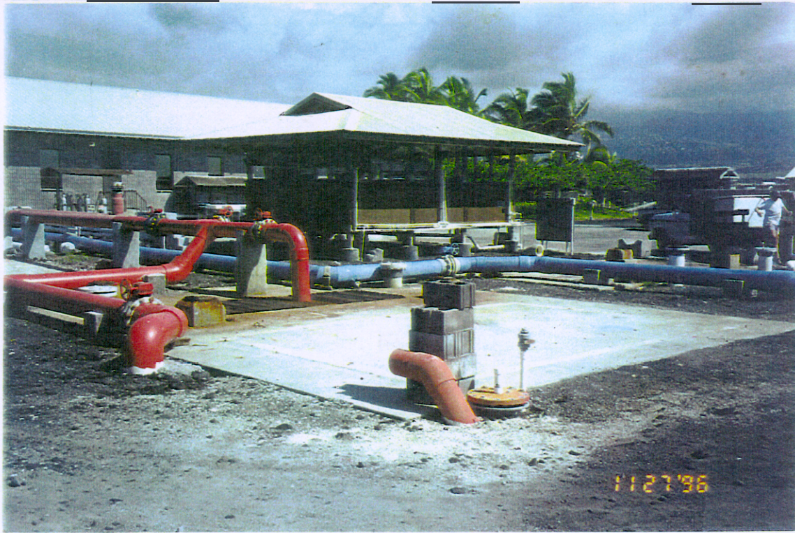
Figure 4-4: Concrete Pad used for Balance of Plant Equipment
