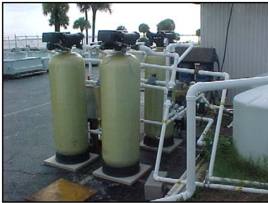
Photo 5 – The two Roughing Filters (Right side).
