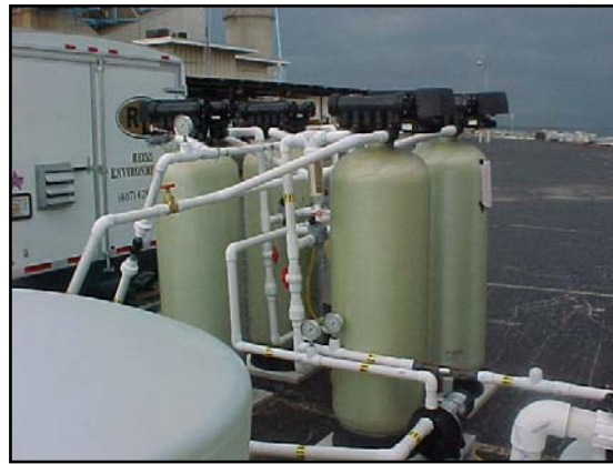
Photo 6 – The two Polishing Filters.
