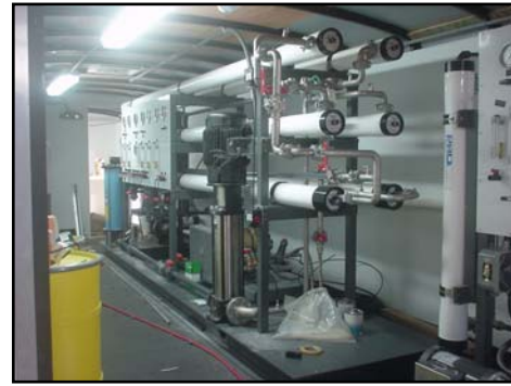
Photo 2 – Seawater RO membrane system.
