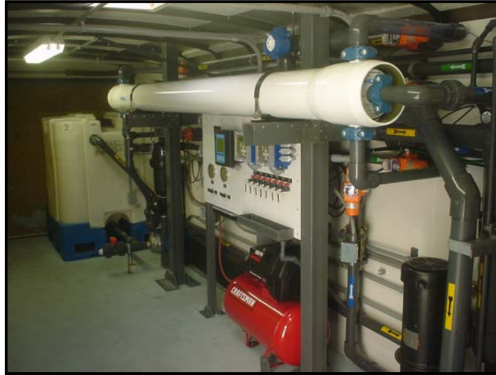
Figure 3-5. Norit Americas Trailer-Mounted UF Pilot Plant.
