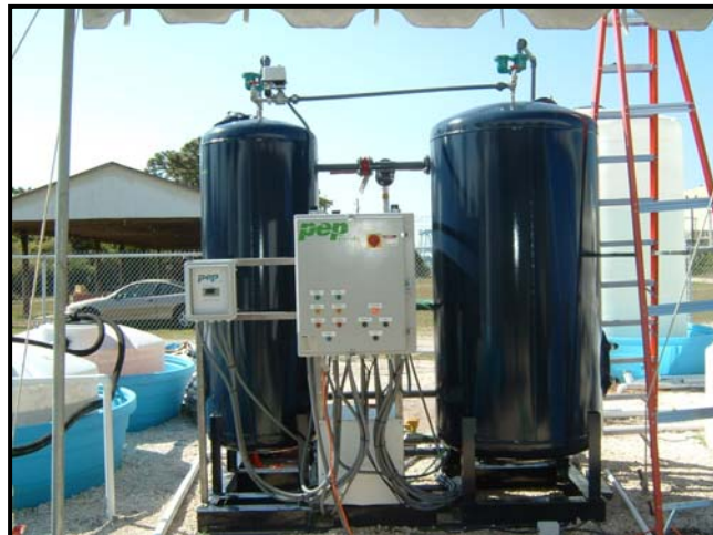
Figure 3-4. Multimedia Filtration Pilot Unit – West Coast Site.
