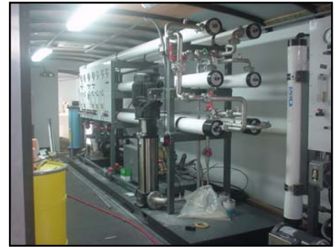
Photo 2 – Seawater RO Membrane System.
