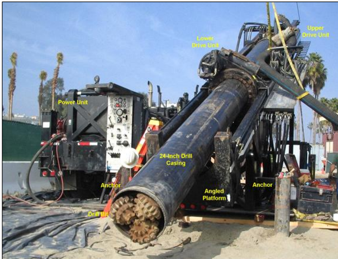
Dual rotary drilling rig (DR-24HD) drilling MWDOC test slant well, Dana Point, California (photo by GEOSCIENCE).
