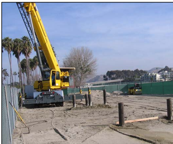
Hollowstem auger rig setting anchors used to stabilize dual rotary drill rig (photo by GEOSCIENCE).
