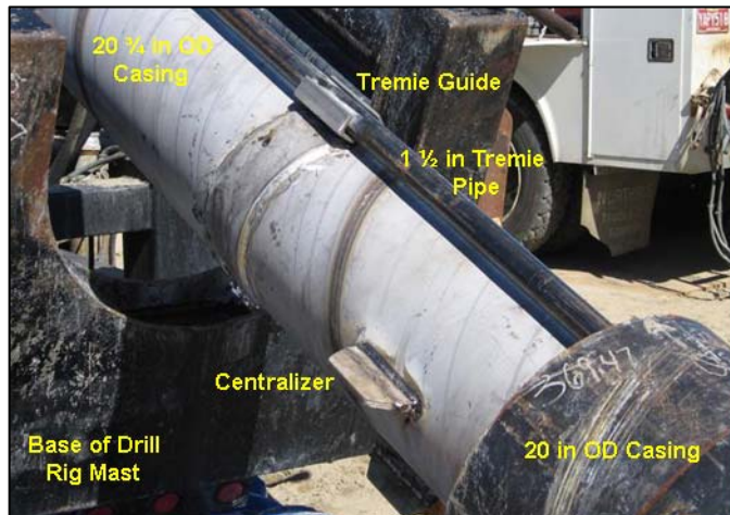
Tremie pipe held in guides attached to top of screen (photo by GEOSCIENCE).
