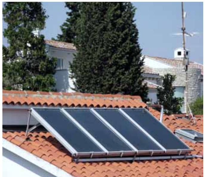
Illustration 4. Solar water heaters on a roof
