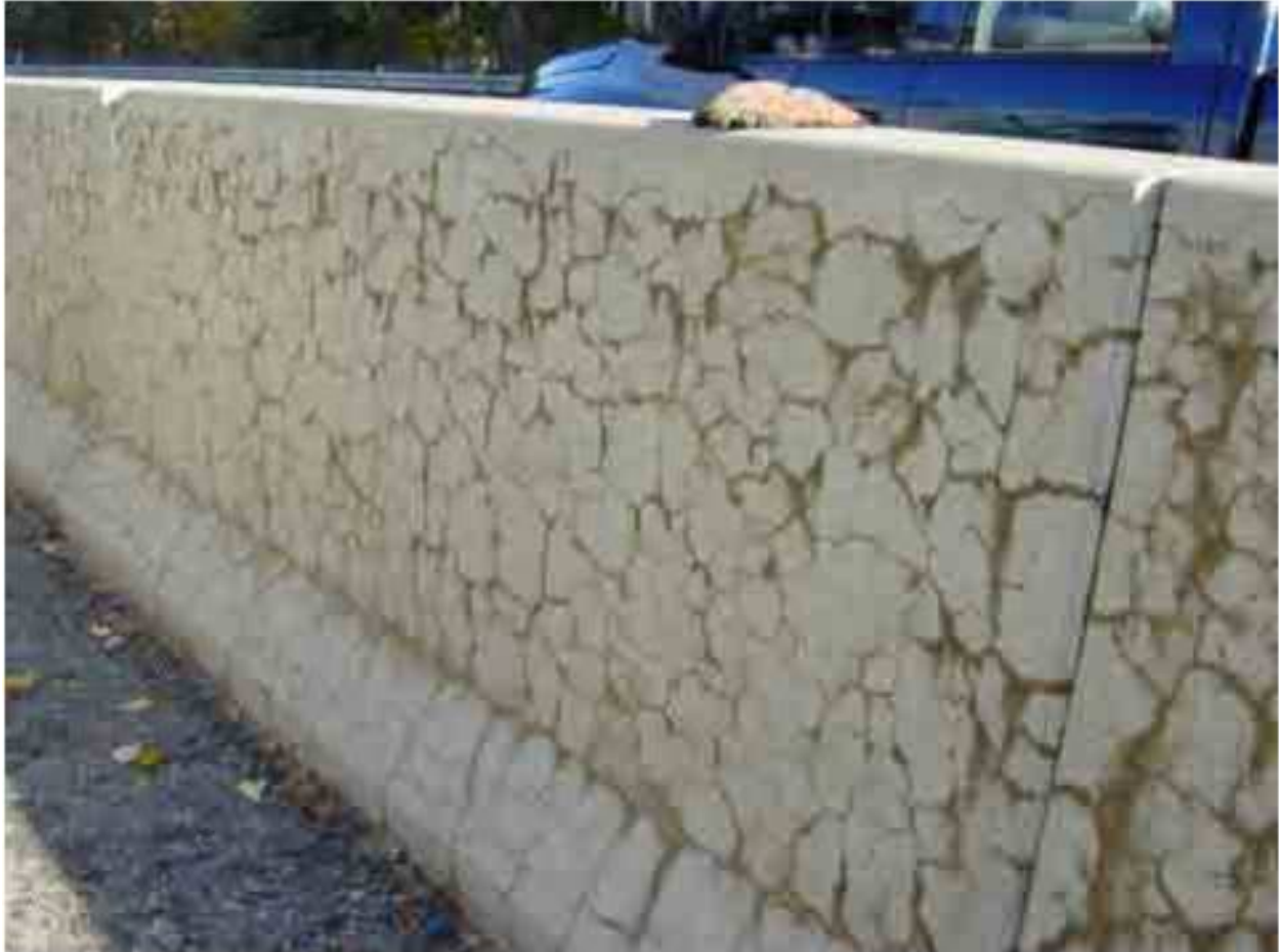
Figure 1 Patterned cracking indicative of ASR-induced degradation (generic example–NOT from nuclear industry)
