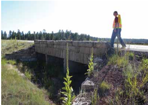
RSAs EXAMINE ROADWAY AND ROADSIDE FEATURES THAT MAY POSE POTENTIAL SAFETY ISSUES.
