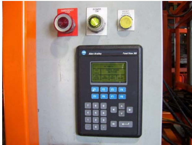
Figure 4. Control panel view.
