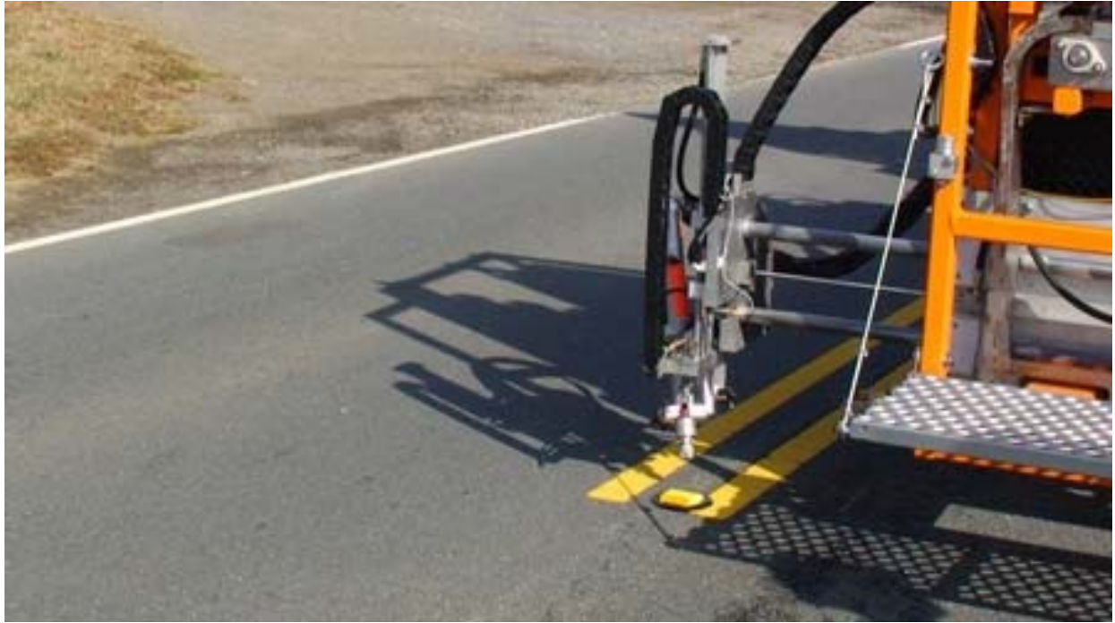
Figure 22. The marker was installed with the right amount of adhesive and force.
