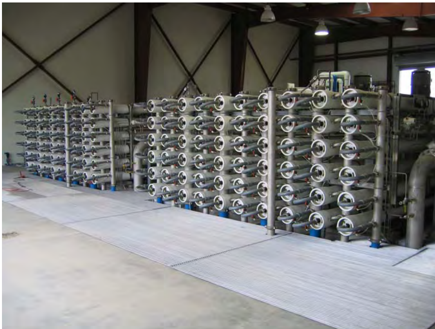
FIGURE 3.8 EMWD PERRIS DESALINATION FACILITY RO MEMBRANES
