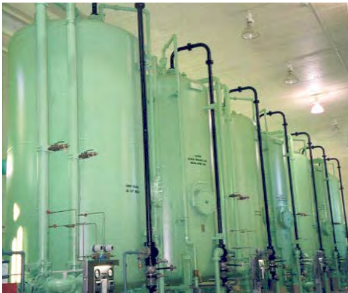
FIGURE 3.2 GAC TOWERS USED IN THE WATER TREATMENT INDUSTRY
