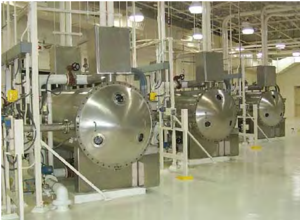
FIGURE 3.5 OZONE CONTACTORS IN CLARK COUNTY, NEVADA
