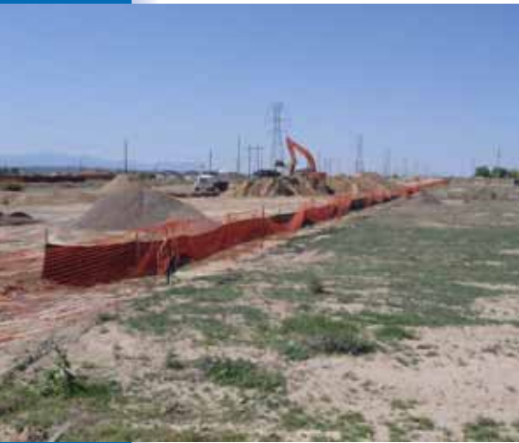
Best management practices would include silt fences to manage erosion during construction.
