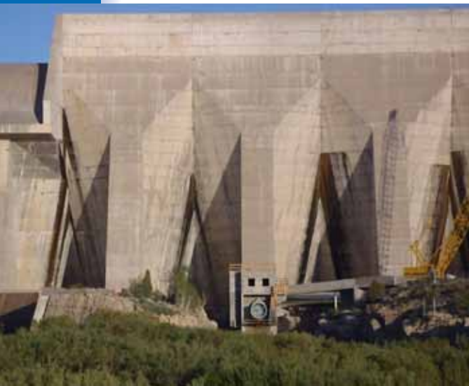
The Interconnect pipeline would connect the existing Pueblo Reservoir south outlet works manifold to the north outlet works shown here.
