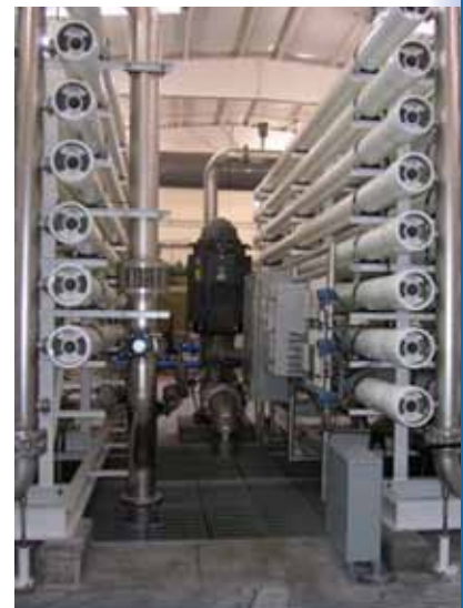
La Junta (regional provider) reverse osmosis water treatment facility.
