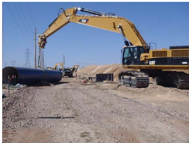
Photo 4-16. Typical construction activities that would cause noise (Southern Delivery System pipeline installation in Pueblo West).
