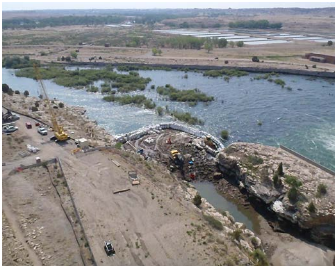
Photo 4-1. Example of construction-related direct effects on a riparian area.
