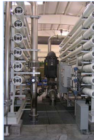
Photo 2-2. Tubular modules and pump at La Junta's existing reverse osmosis water treatment facility.
