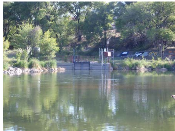
Photo 2-10. AVC supplies under the River South Alternative would be diverted near the St. Charles Mesa intake structure on the Arkansas River.
