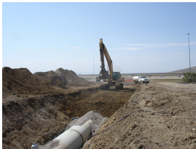
Photo 1-3. The AVC would be a buried pipeline, similar to the one shown in this photo, and would convey water from Pueblo Reservoir east to Lamar.
