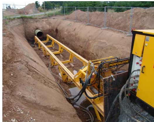
Photo 2-11. Trenchless construction techniques could be used to avoid disturbing major roadways, streams, and other resources.
