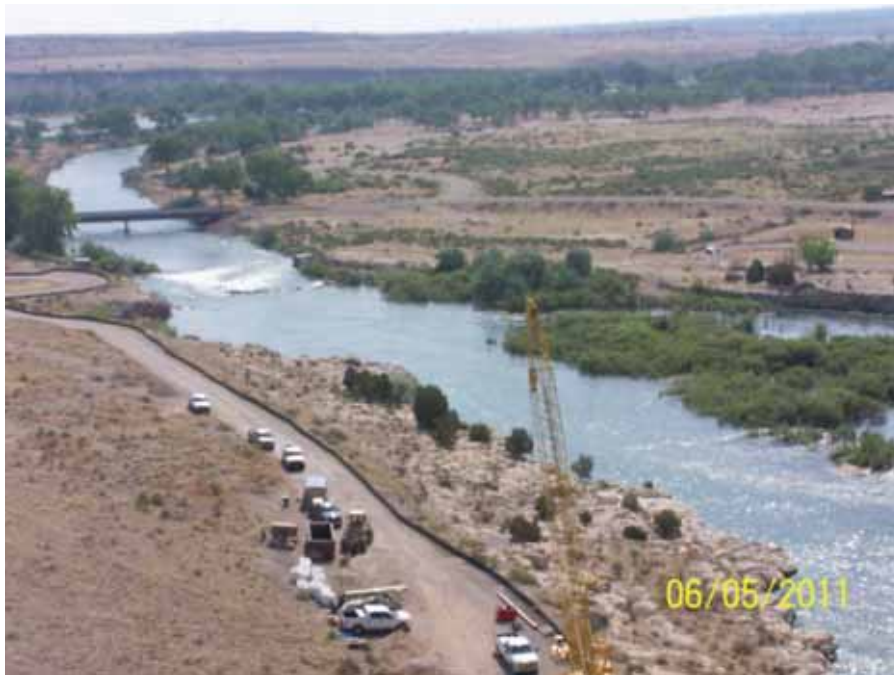
Photo 4 - AVC Pueblo Dam Outlet Works Interconnect site. Photo taken from top of Pueblo Dam, looking east. Pipeline crossing approximately 150 feet upstream of Juniper Road bridge. Photo by Rodney Barthel
