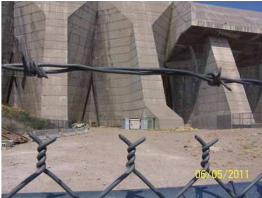
Photo 6 - Pueblo Dam toe Electrical Switchgear located near abutment No.7 on south side of dam. Photo by Rodney Barthel
