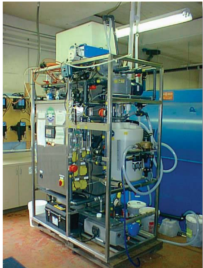
One of the verified UF technologies
