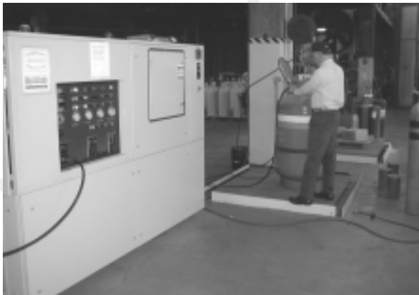
Technician connecting hose to a halon storage cylinder from a halon recycling unit operated in accordance with NFPA standards. EPA regulations prohibit disposal of halon except by sending it for recycling to a recycler operating in accordance with NFPA standards – or by arranging for its destruction via approved processes. Photo courtesy of U.S. DOD/DLA ODS Reserve.
