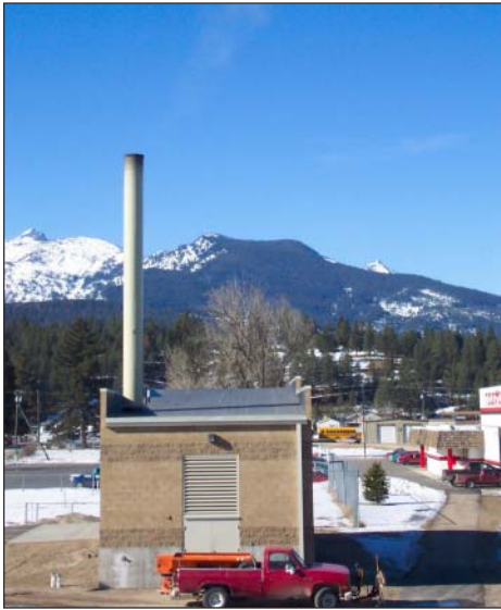
This biomass boiler provides heat to the school in Darby, Montana. Emissions are very low from this type of boiler. (Photo by U.S. Forest Service)
