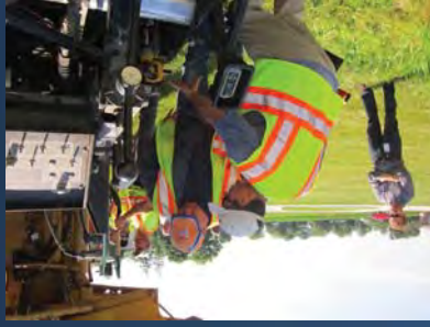
This Indiana demonstration project provided the opportunity for on-site explanation for improving quality of the edge
