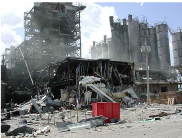
Damage from an explosion and fire at a manufacturing facility in 2004. Vinyl chloride monomer, a regulated substance under the Risk Management Program, fueled the explosion and fire, which caused evacuation of the nearby community. (Photo courtesy U.S. Chemical Safety and Hazard Investigation Board)
