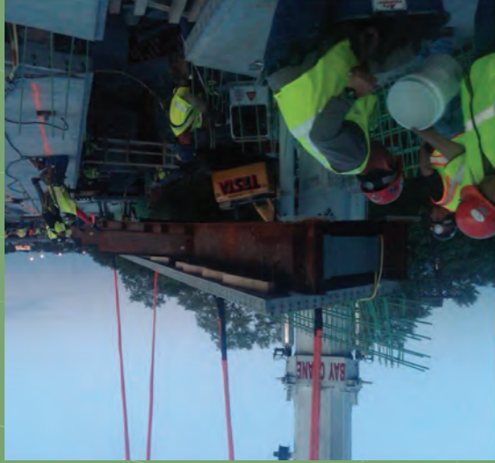
MassDOT Fast 14 Project replaced fourteen bridge superstructures in one construction season using PBES.
