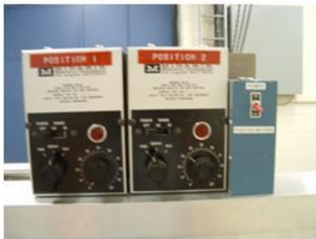
Chamber alignment controls 300 kV range
