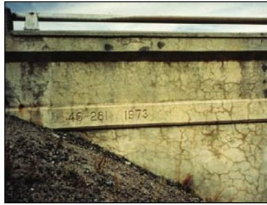
Figure 6. Surface discoloration in a bridge structure caused by ASR.
