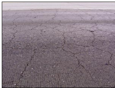
Figure 2. Map cracking in a section of pavement on Interstate 84 near Mountain Home, ID.
