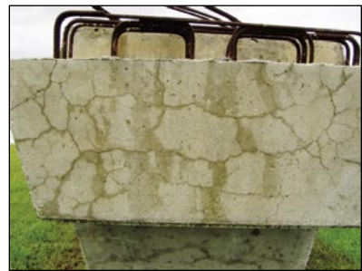
Figure 4. Concrete girder treated for ASR in Corpus Christi, TX.
