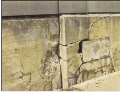
Figure 5. Misalignment of adjacent sections of a parapet wall on a highway bridge due to ASR-induced expansion. (2)
