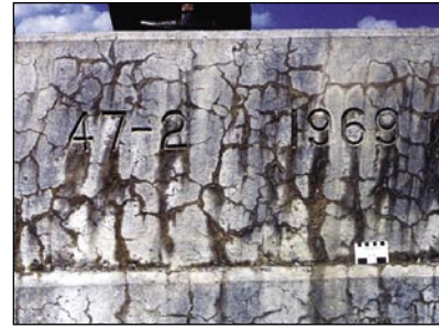
Figure 7. Concrete structure showing discoloration, or "gel staining," around cracks.
