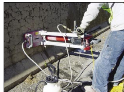
Figure 8. Core extraction from a concrete barrier along State Highway 2 near Leominster, MA.
