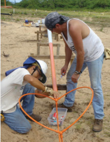
Figure 4. Dean Takamatsu and John Lowe assemble new corrosion-resistant antennas for NIST time and frequency radio station WWVH in Kauai, Hawaii.
