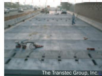
A 38-m (124-ft) section of post-tensioned, precast pavement in place on the Caltrans I-10 installation.
