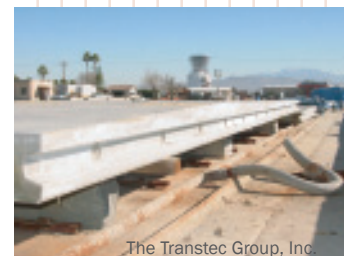
In the California I-10 demonstration, the panels used a crown shape that tapers from 330 mm (13 in.) at the high point to 250 mm (10 in.) at the ends.
