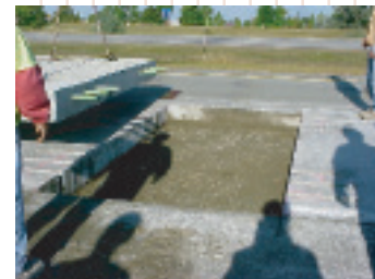
Single-panel replacements were installed in lieu of full-depth patches on Michigan's I-94.
