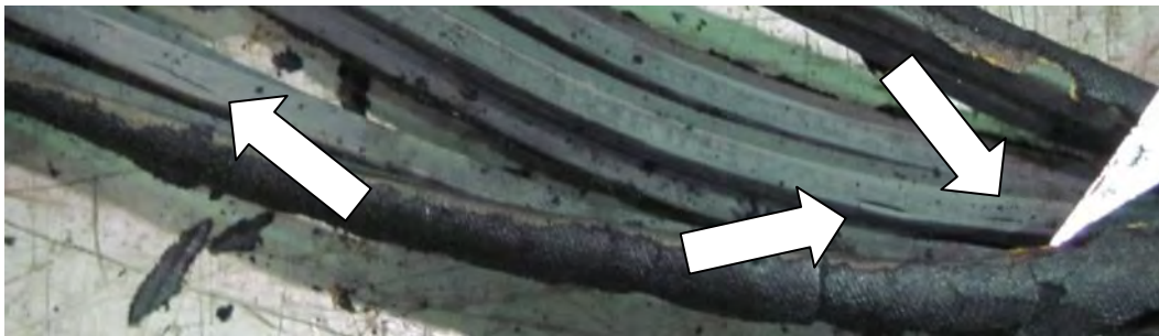
Figure 7.21: Longitudinal cracking found along the conductors of Item E
