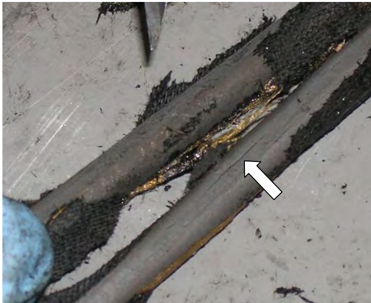
Figure 7.38: Longitudinal cracking observed during the post-test analysis is visible as a dark line running along the right hand conductor near the center of the photo.
