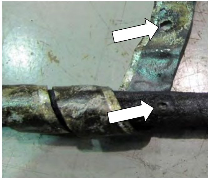
Figure 7.16: Hole in the conductor insulation corresponding to the hole found in the zinc wrap.
