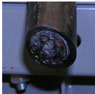
Figure 7.40: Liquid observed from cut end of thermal response cable during Test K4.
