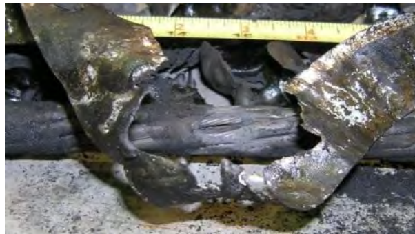
Figure 7.47: Removal of the zinc wrap and charred insulation material reveal the bare copper conductors.
