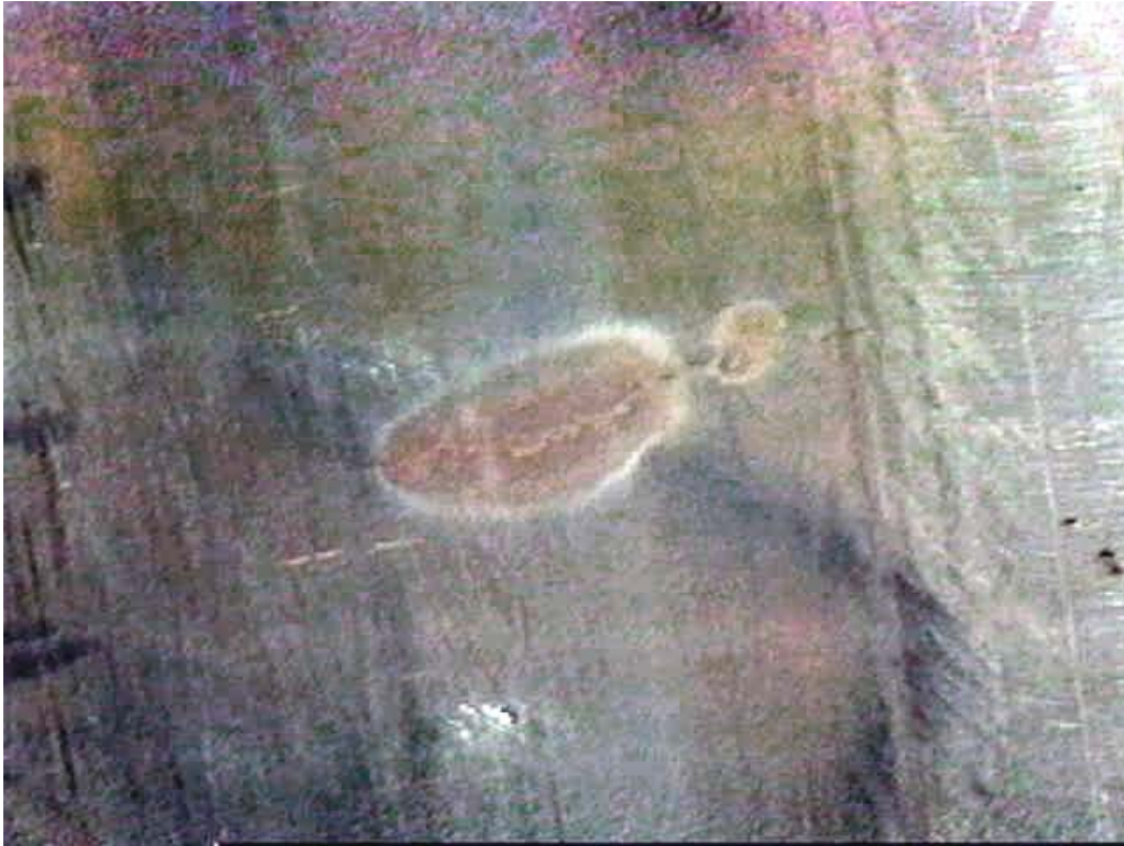
Figure 6.6 Stress Corrosion Crack Through Stainless Steel Made More Visible by Oxide Decoration
