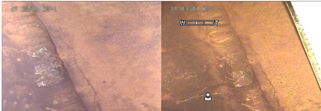
Figure 6.3 A Crack Before (left image) and After (right image) Cleaning Loose Oxide Layer from Surface
