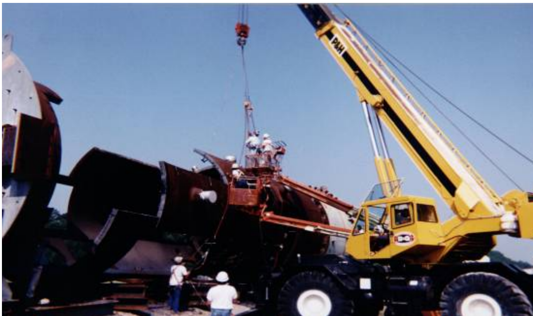
Figure 3.9 River Bend Unit 2 RPV During Disassembly
