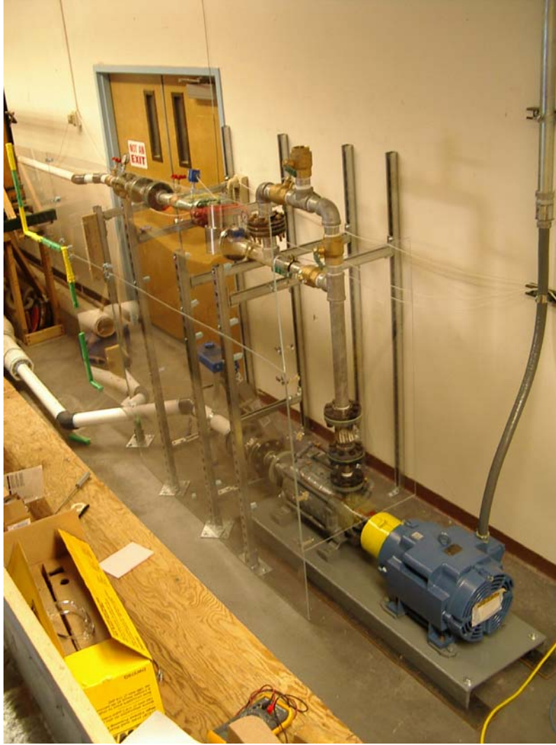
Figure 2-2. Photograph of the Test Loop (Excluding the Flume)
