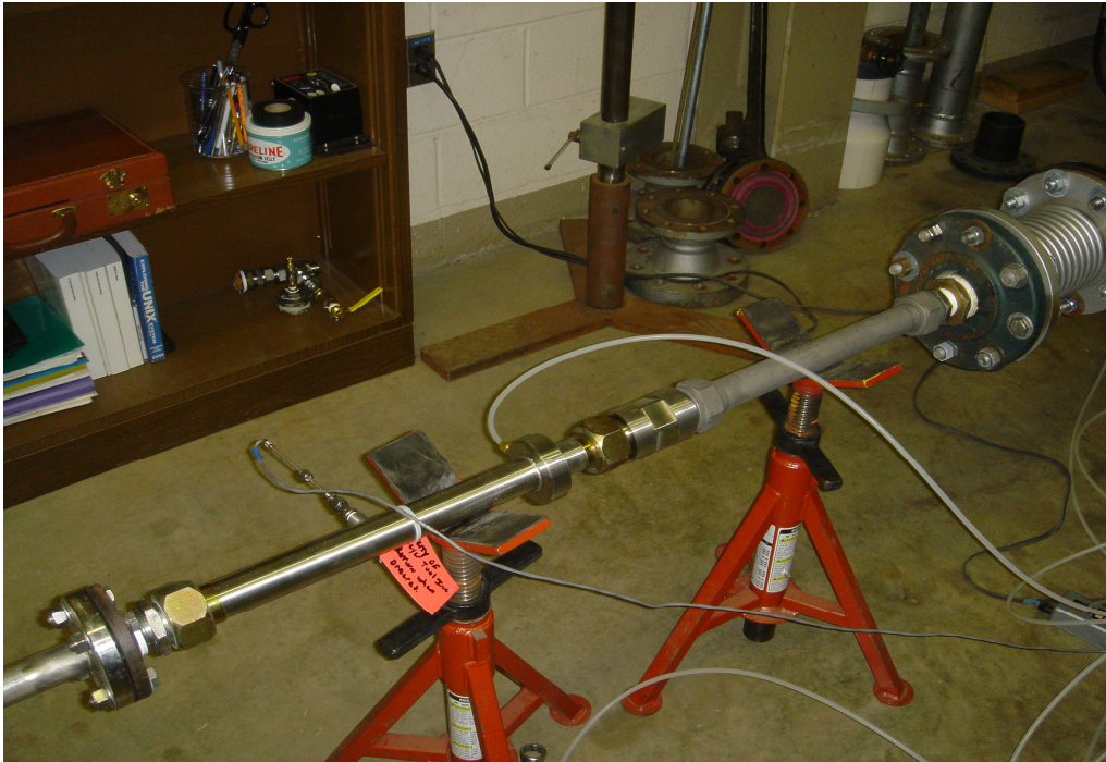
Figure 1. Photograph of the flow meter installation.
