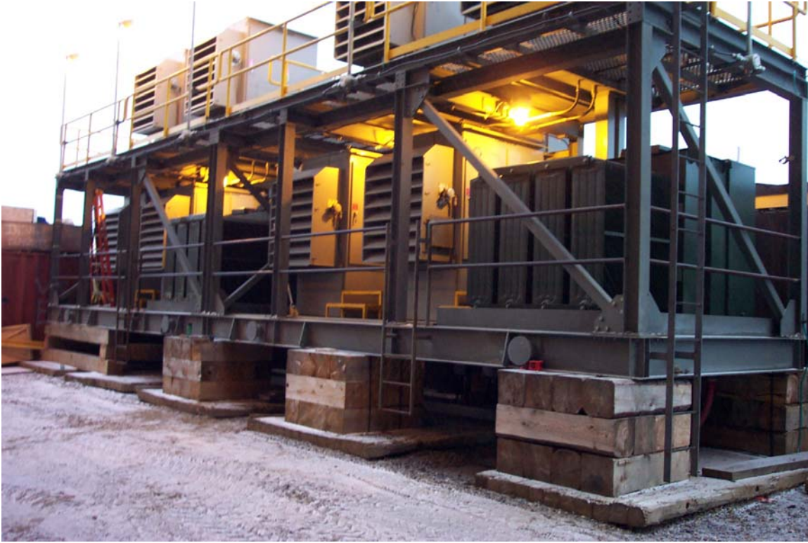
Figure 2.3: Load Bank and Supports
