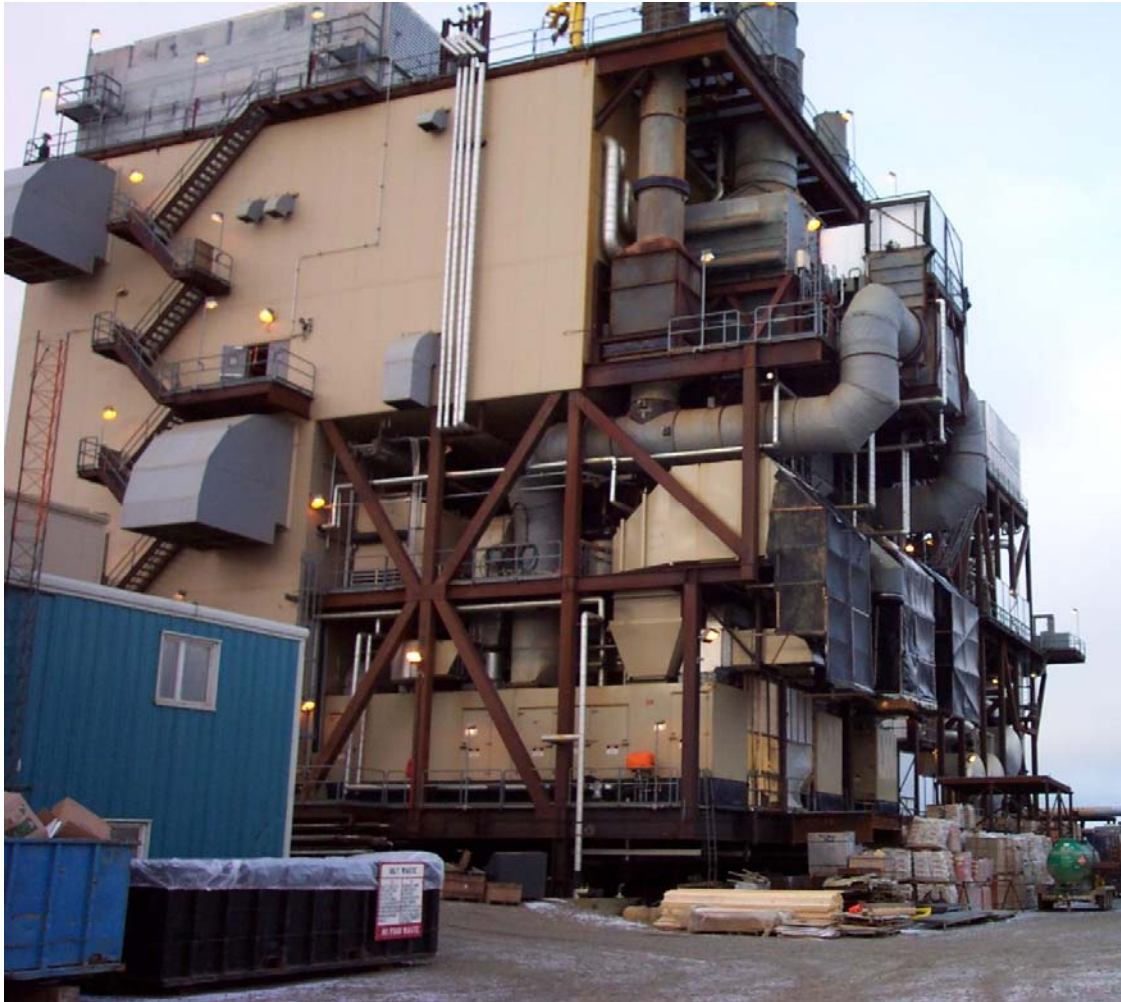
Figure 2.2b: South Process Module
