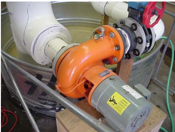
Figure A.11. 5-hp motor at the base of the vertical test section of the hydraulic loop.
