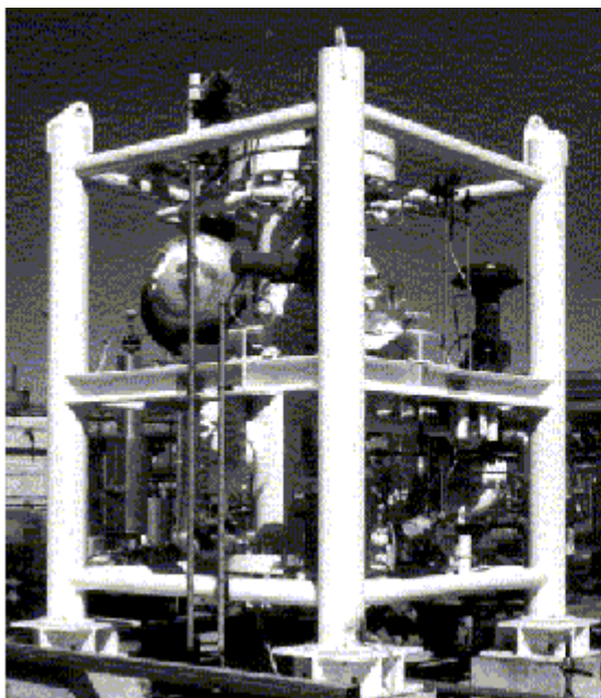
Fig.3.38. Prototype installed in field
