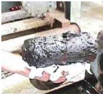
Figure 5.2: An asphaltene plug removed from a pipeline 5 .
