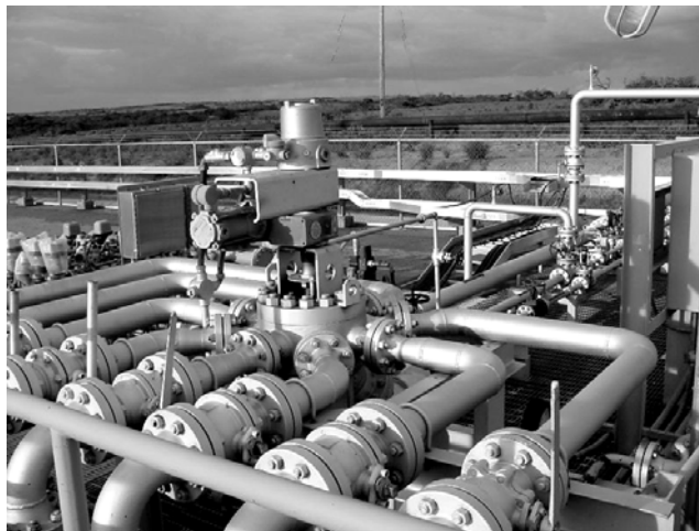
Figure 9.3: A multi-port valve switches production of each well from the main line to the multiphase flow meter.
