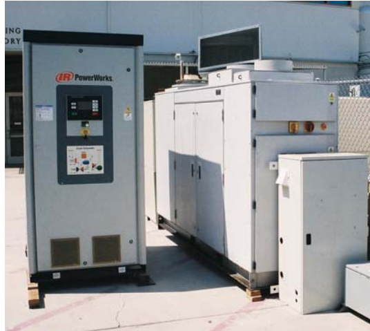
Figure 3. 80 kW Bowman microturbine received from Southern California Edison
