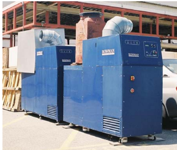
Figure 4. 35kW and 60 kW Bowman microturbines received from Southern California Edison.
